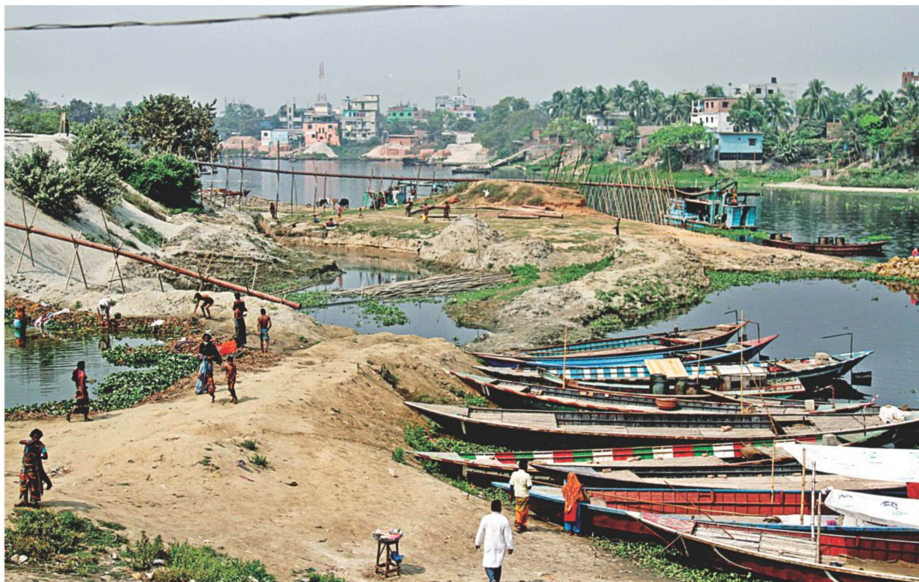
Encroachers and traders have created a strip of land in the Turag river by dumping earth so that they can extract and transport away sand easily. Though Bangladesh Inland Water Transport Authority (BIWTA) conducted a drive there less than a year ago to ensure smooth flow of water, it did not remove all the earth, rendering the effort fruitless. Similar incomplete drives are seen elsewhere too. The photo was taken at Sinnirtek near the capital's Mirpur beribadh yesterday.
