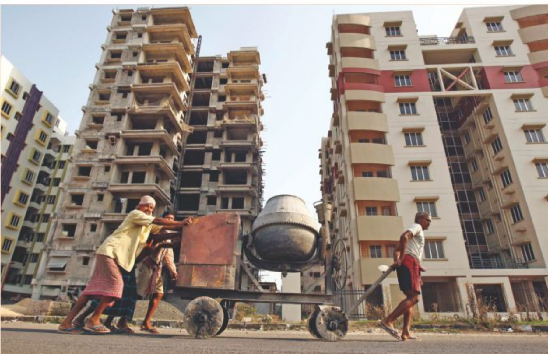
Labourers move a concrete mixer past an under-construction site of residential buildings in Kolkata yesterday.
