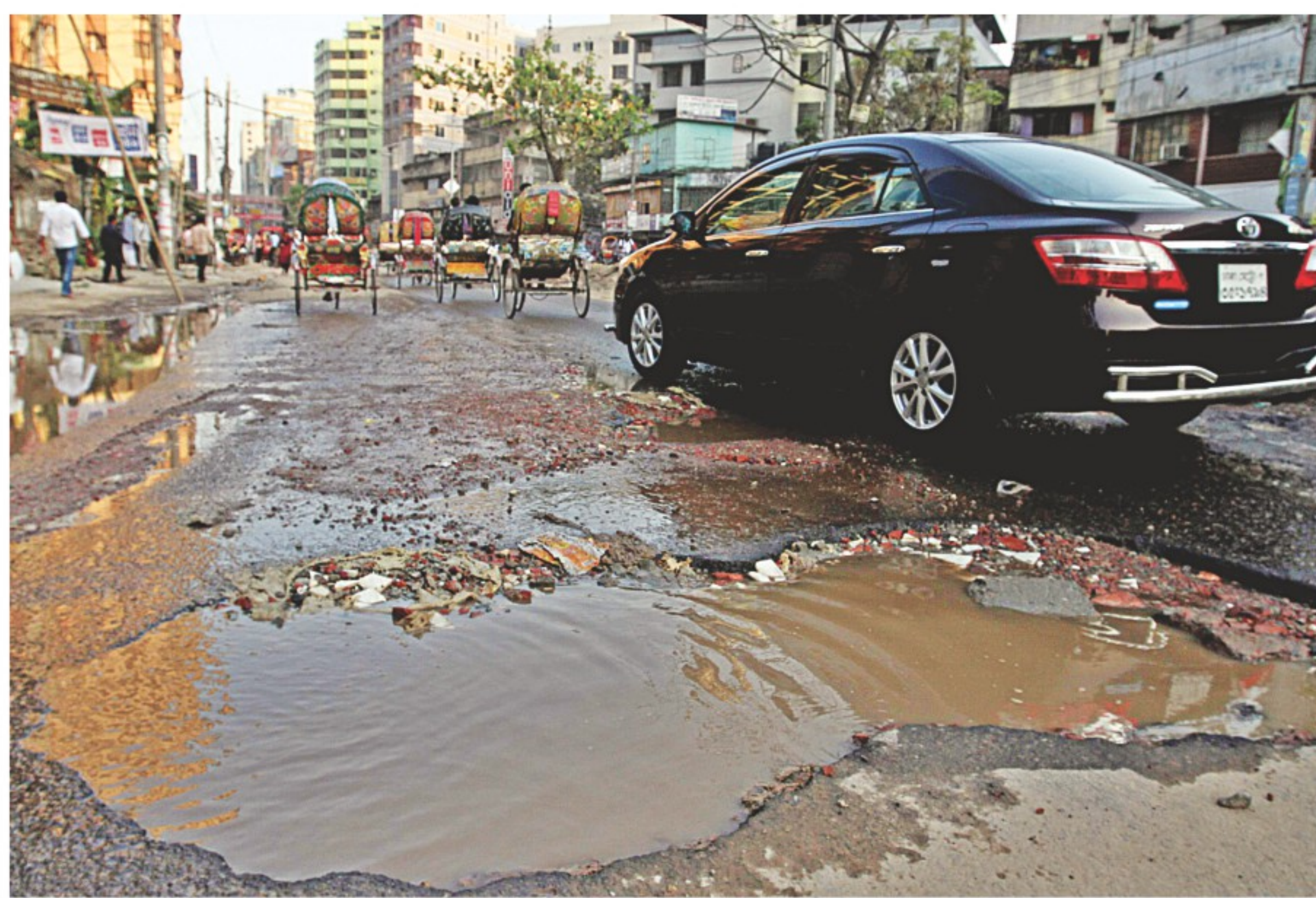
A large crater lies across the outer circular road between Siddheshwari and Mouchak of the capital, hampering vehicular movement for over half a month. The photo was taken yesterday.
