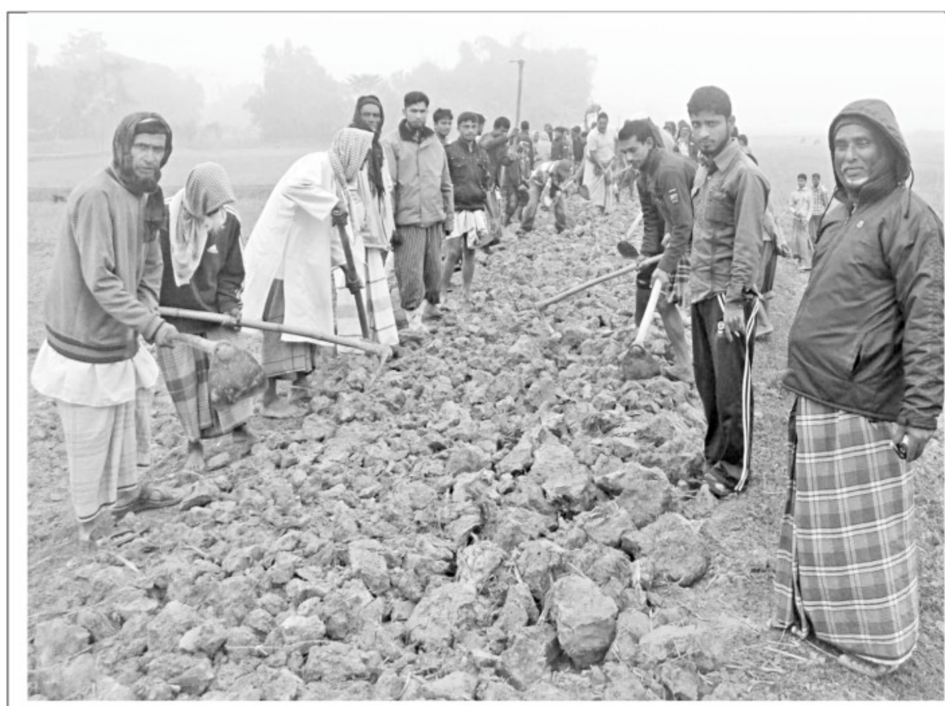
People of Protapi village in Komolganj upazila of Moulvibazar join hands to renovate the road in their area as the authorities concerned did not take any step in this regard despite several pleas in the last two years.
