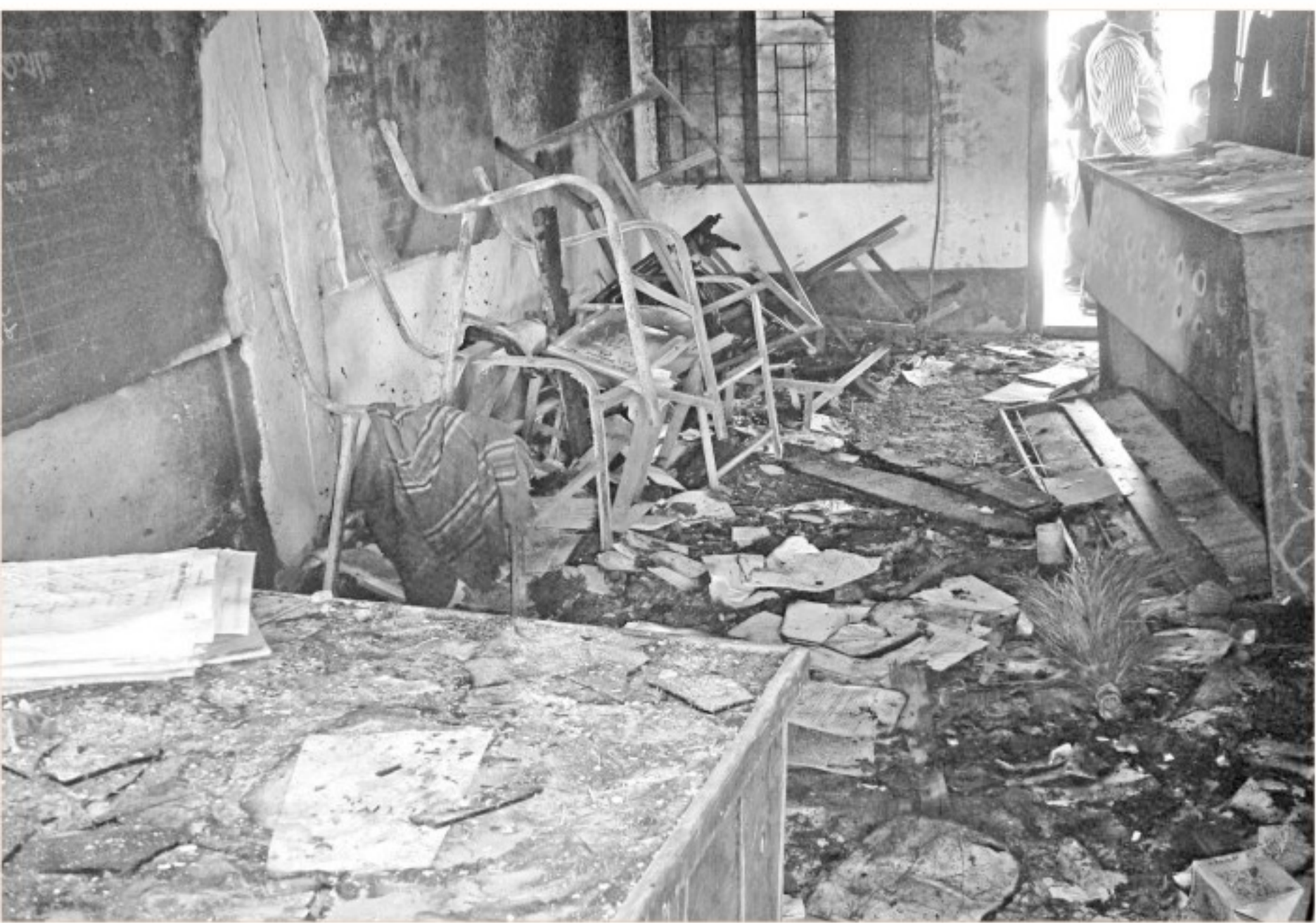
The remains of the furniture of Mamunshia Govt Primary School in Kotchandpur of Jhenidah after criminals torched the school ahead of the January 5 polls. Top, destroyed furniture at Fulbari Govt Primary School in the same upazila. Bottom, Marks of the blaze at Charghat-Bagha Shyampur Govt Primary School in Rajshahi. All the schools were supposed to be polling centres.
