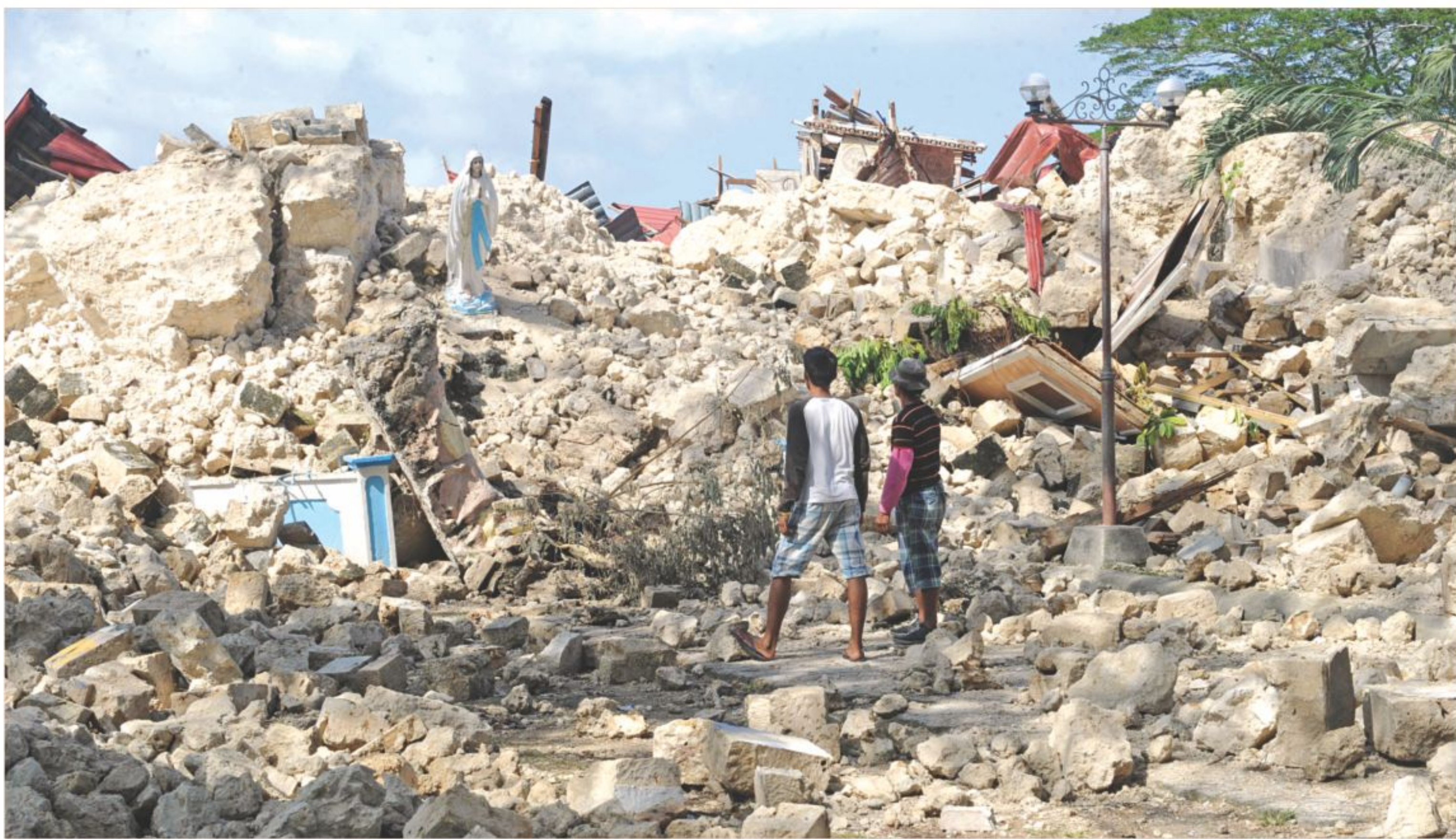
Philippine residents look at the ruins of the historic Holy Cross Parish Church in Maribojoc town in the central Philippine island of Bohol, that was damaged during the 7.1 magnitude quake that hit the area on Tuesday, leaving over 180 dead. Philippine rescuers yesterday called off the search for survivors.
