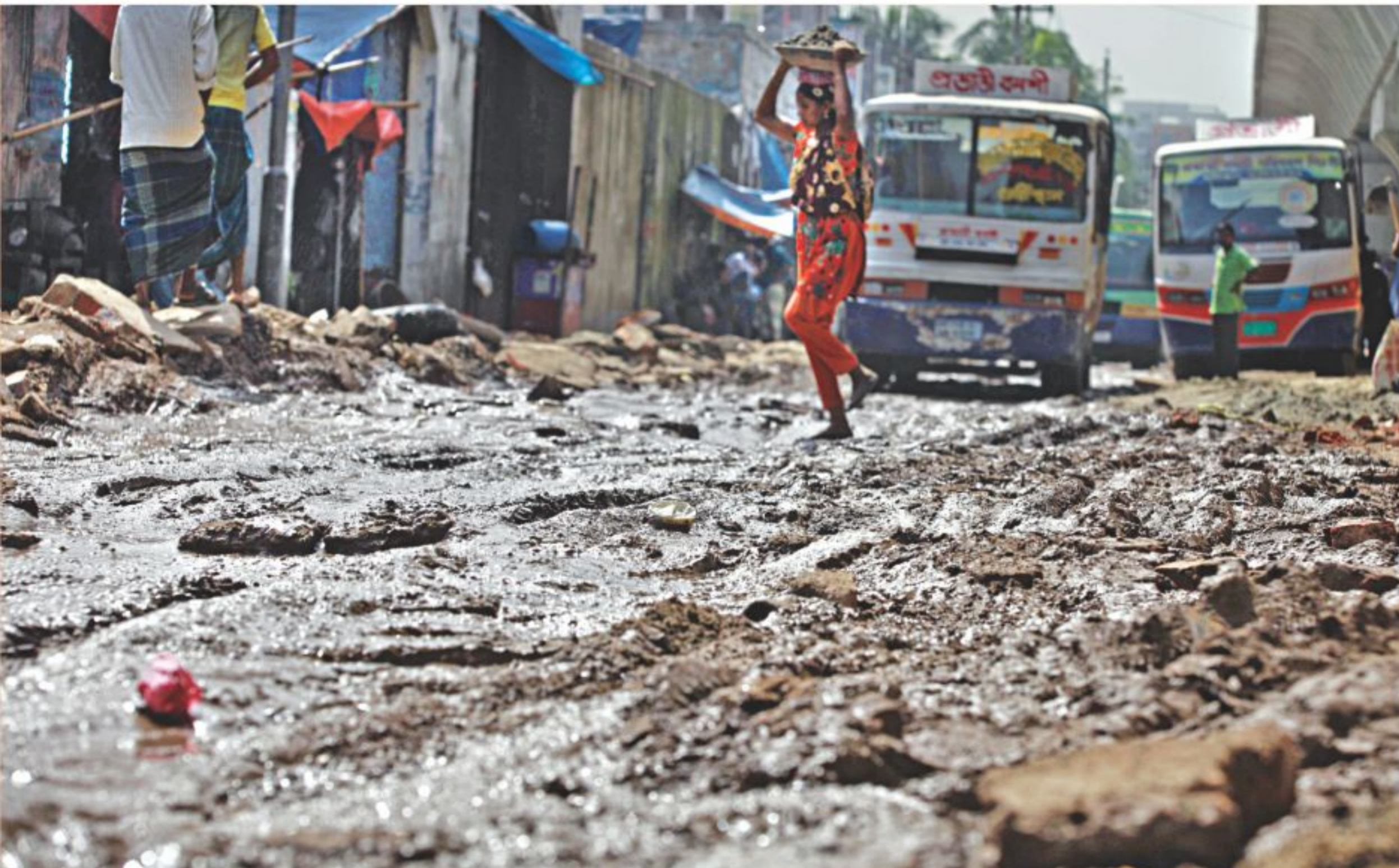
A road in Phulbaria, Gulistan, in Dhaka, is in a pathetic condition. When it rains, the road becomes muddy, making travelling through it a terrible experience for pedestrians and drivers. PHOTO: STAR
