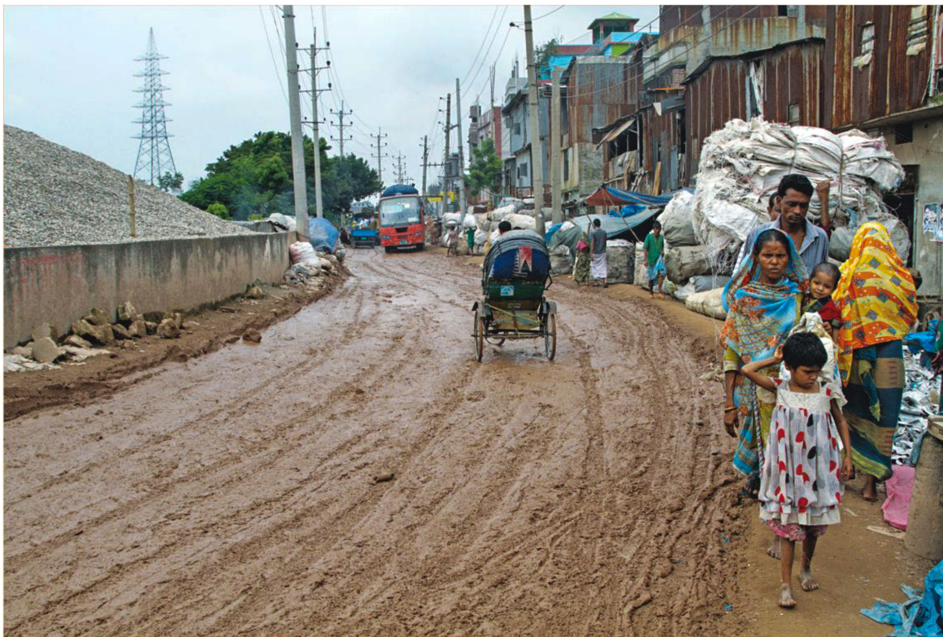
This pothole-riddled, muddied road in Kamalbagh Beribadh area in the capital's Lalbagh has been like this for around six years and the situation worsens after rains. The suffering locals allege that the authorities concerned did not take any step for repairs despite repeated requests.
