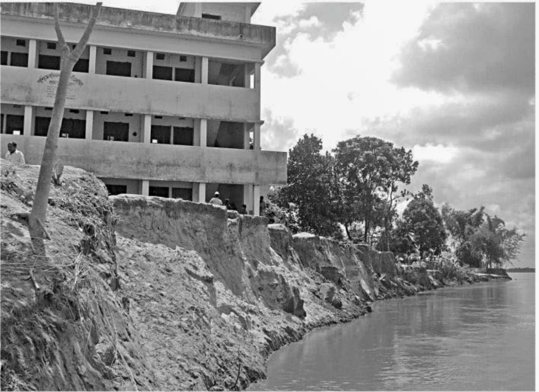
Dhaniram community centre-cum flood shelter in Phulbari upazila of Kurigram district is on the verge of collapse into the Dharla as erosion by the river has taken a serious turn in the area.
