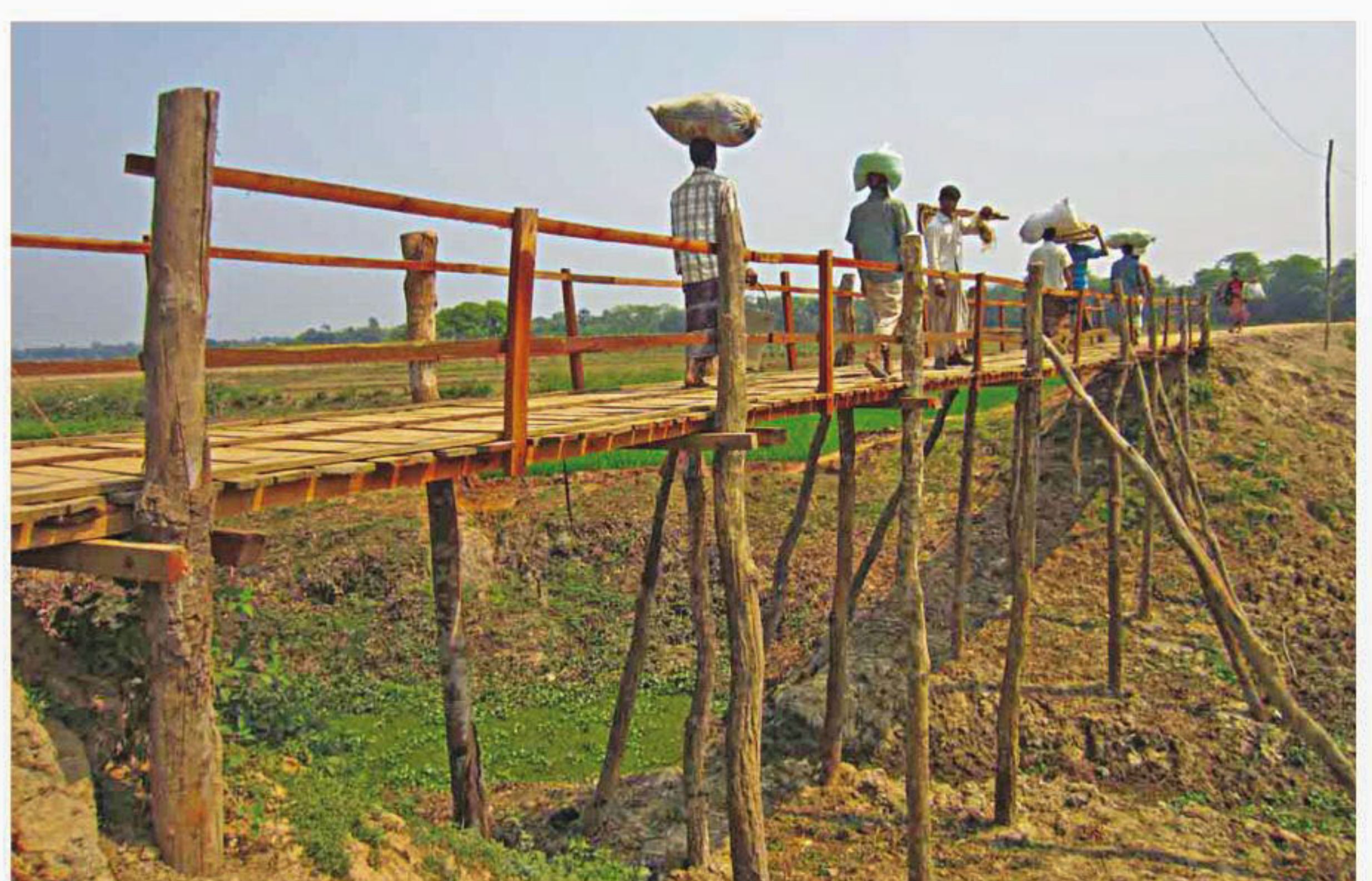
Villagers carrying their loads on head walk across the Marta-Martar Char bridge towards the highway leading to Gazipur district town as the wooden structure is unfit for heavy vehicles, even rickshaws. Around 20,000 people of different villages in Sreepur upazila, who use this bridge, have long been demanding its replacement with a concrete one. The photo was taken recently.
