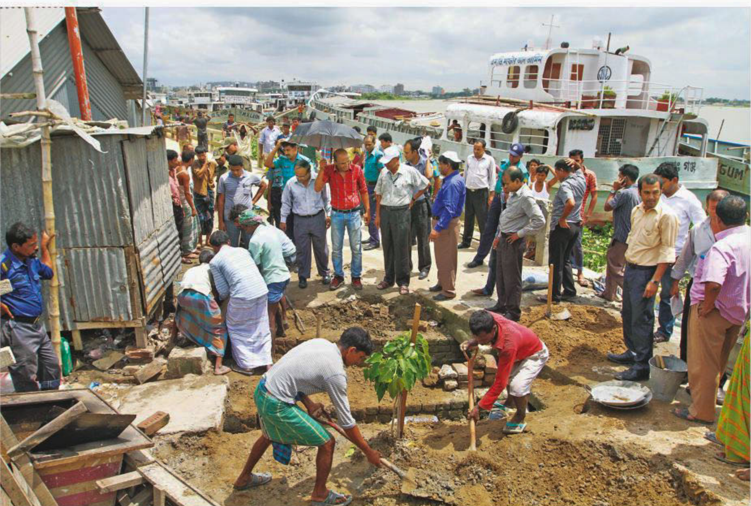
The workers of Bangladesh Inland Water Transport Authority (BIWTA) seal a drain, through which factory wastes used to stream into the river Buriganga, at Gabtoli on the outskirts of the capital yesterday. PHOTO: AMRAN HOSSAIN
