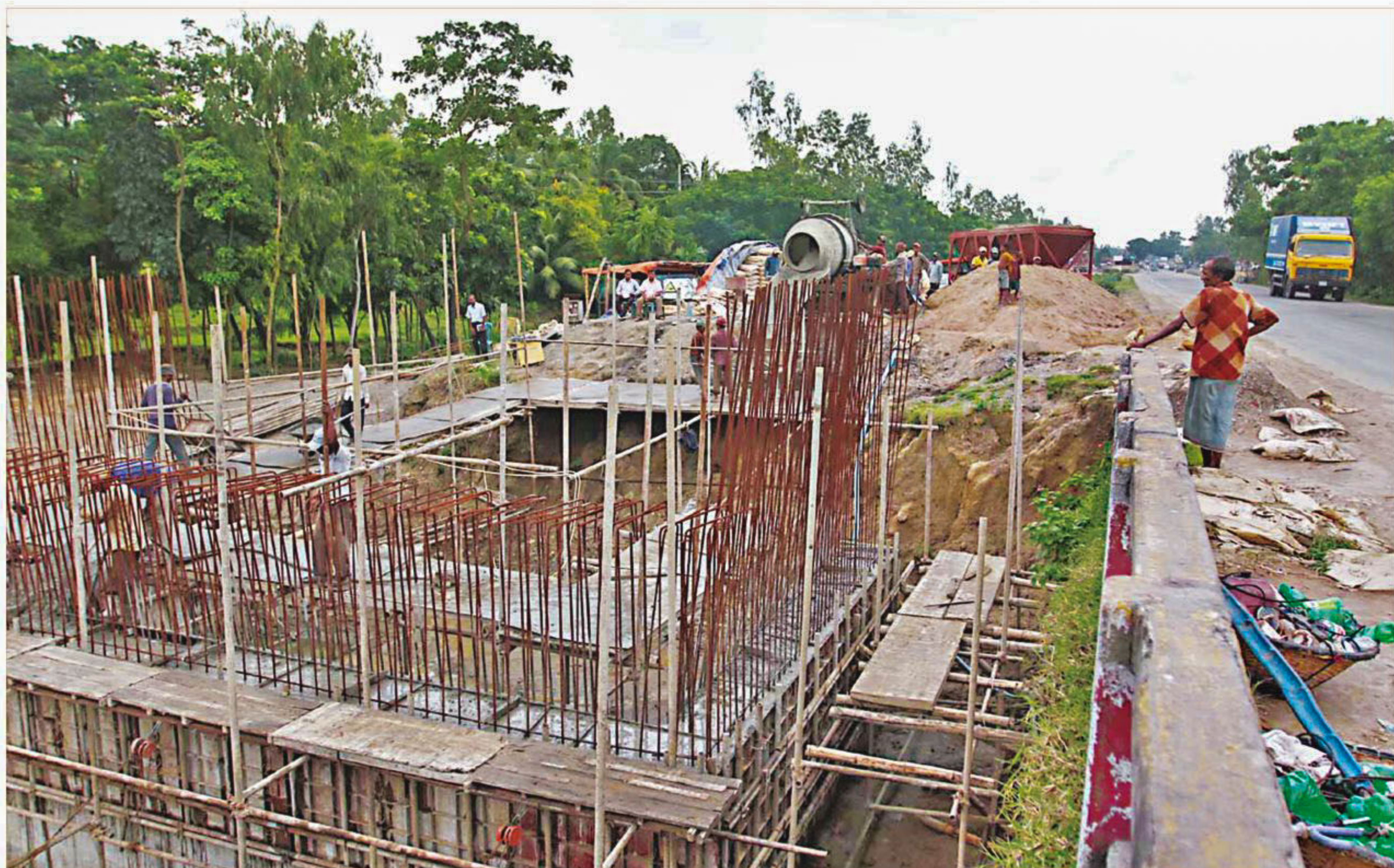
This photo taken about six months ago shows a culvert being built at Sitakunda in Chittagong as part of the Dhaka-Chittagong highway dual-carriageway project. The construction work has not progressed much there since.
