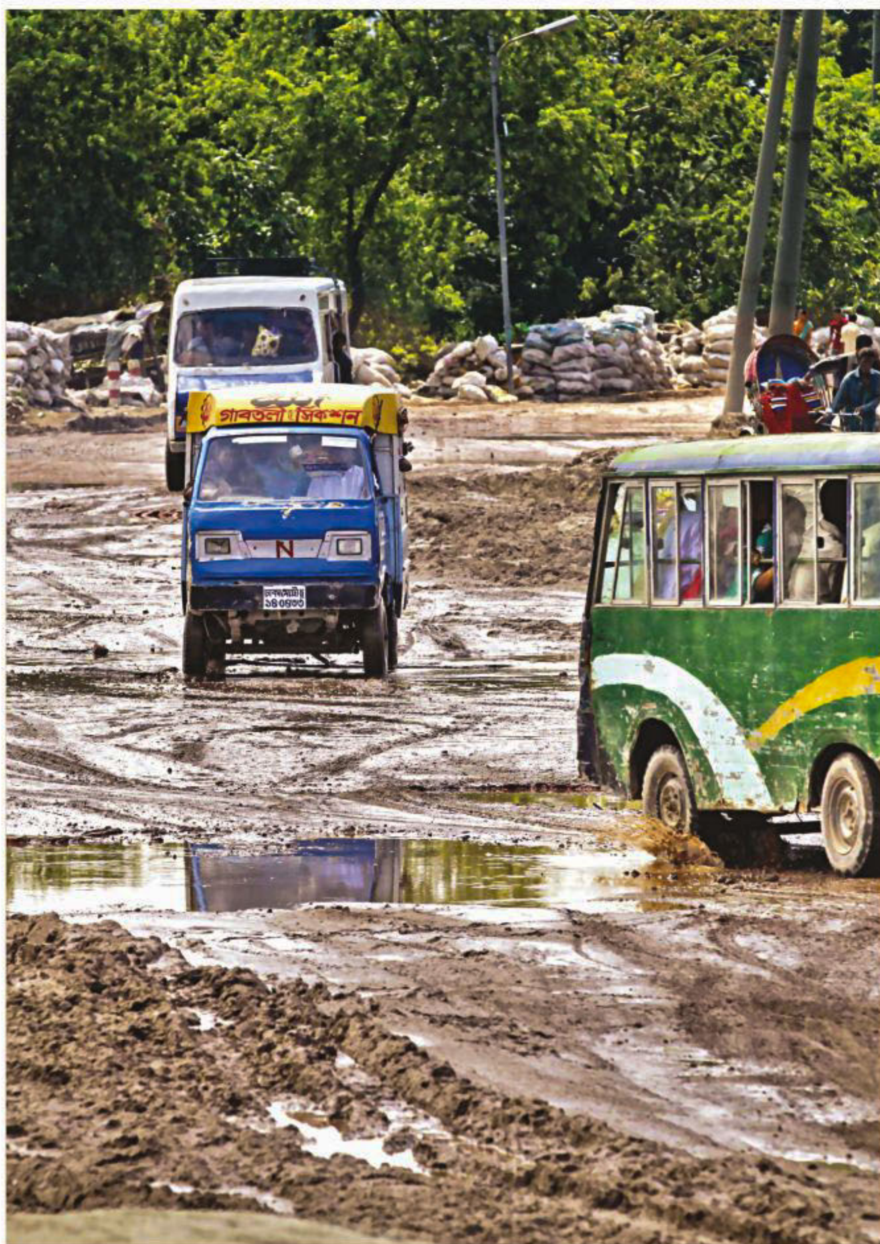
Vehicles operate on the Gabtoli-Babubazar link road, which has long been damaged, muddy and potholed. Its condition gets worse even after a light rain. The photo was taken yesterday.
