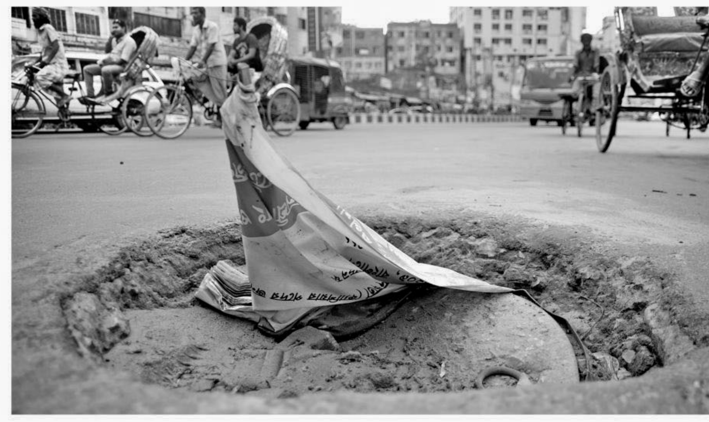
This manhole, lying below the layer of tarmac in the capital's Arambagh, is lost from view whenever rainwater inundates the road, causing frequent accidents. The photo was taken recently. PHOTO: STAR
