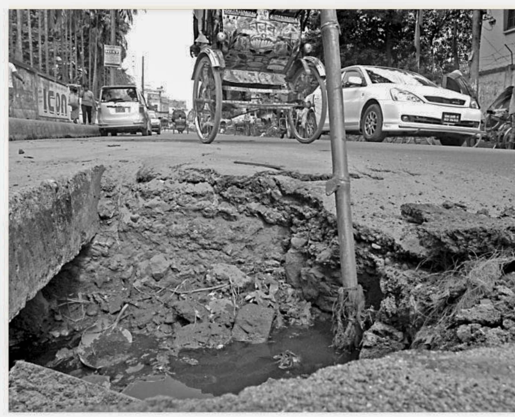
PHOTO: PALASH KHAN This manhole without its lid on the road in front of Tuberculosis Control and Training Institute in Chankharpool of the capital may cause accidents at any time. The photo was taken yesterday.
