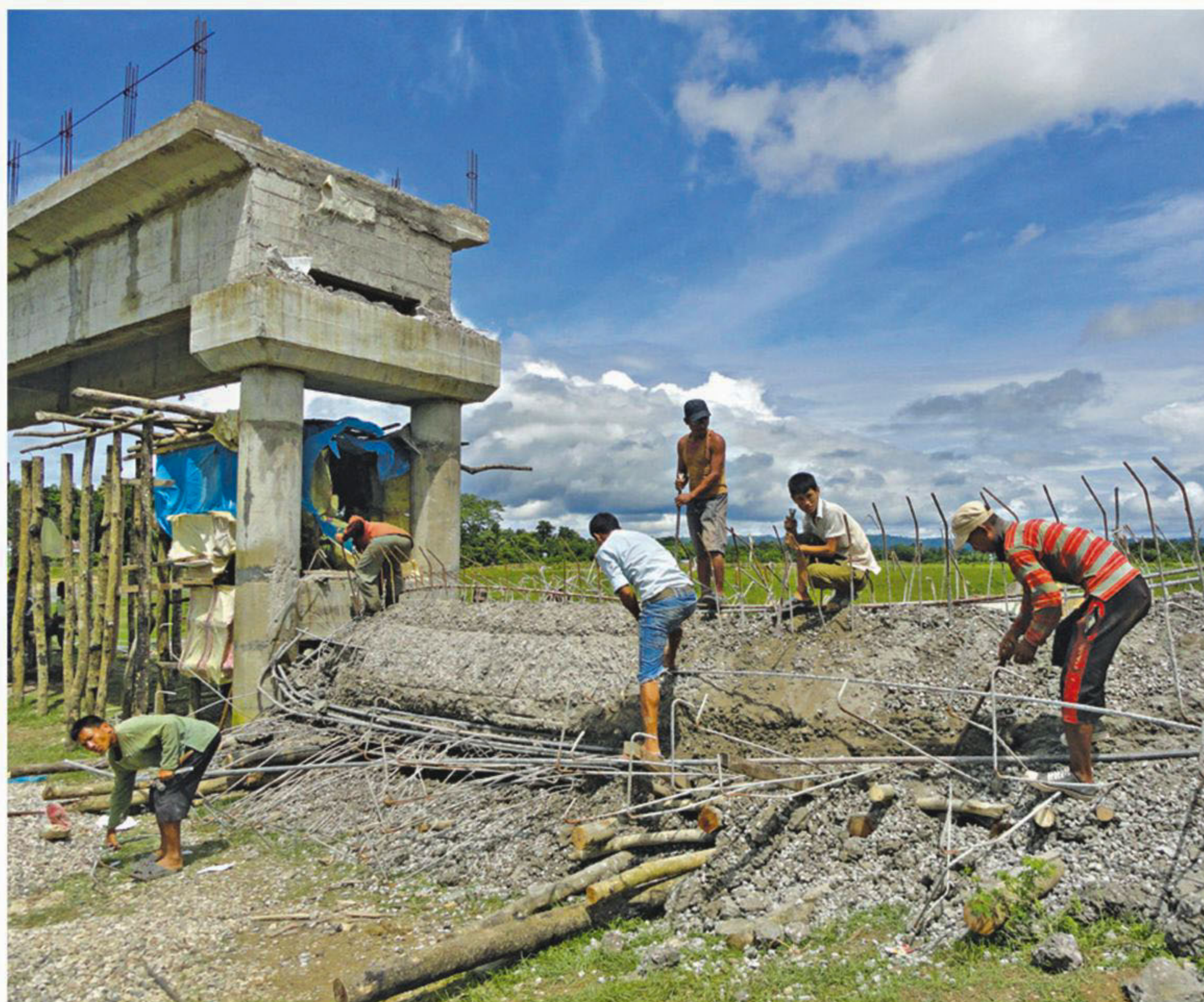
Workers removing rubble yesterday after an under-construction bridge on the Myne river in Khagrachhari collapsed on Tuesday night.
