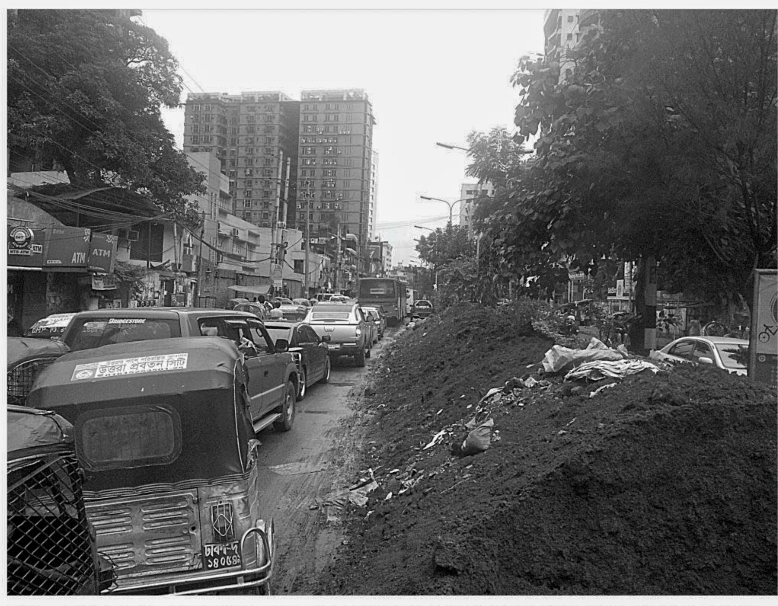
Soil dug out from the New Eskaton Road, where a flyover is being built, is left on the fast lane of the extremely busy street, making the usual gridlock even worse ahead of Eid. The photo was taken yesterday. PHOTO: STAR
