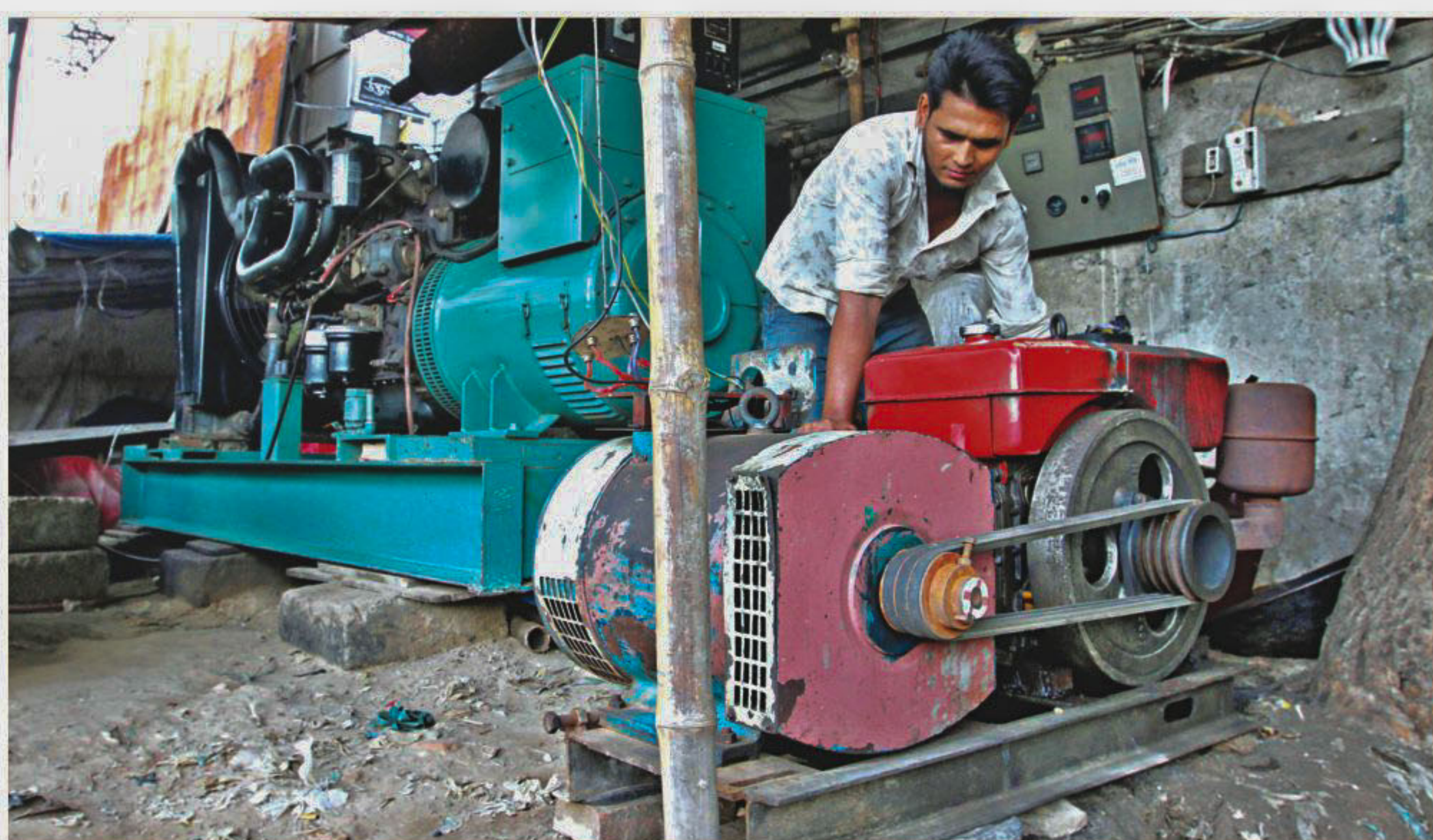
Small generators like these have been set up by traders of markets in the capital so that power supply is uninterrupted during the pre-Eid shopping period. The generators in the photo, taken yesterday, were set up by traders of different markets in Sadarghat area.
