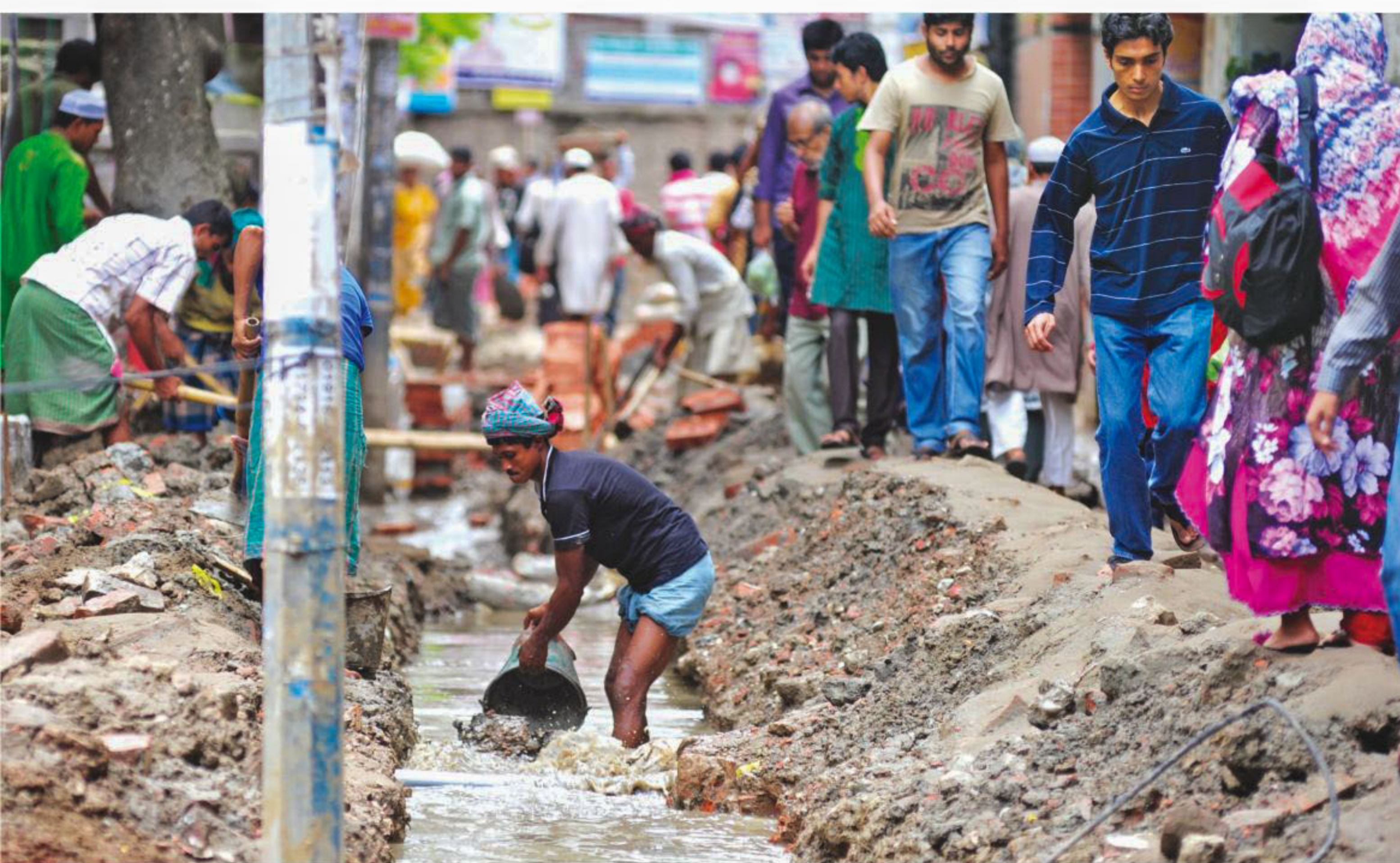
A trench dug for installing utility lines on the capital's Malibagh Bazar Road, which is already in a bad shape, has made life for locals and commuters difficult. The photo was taken on Friday.
