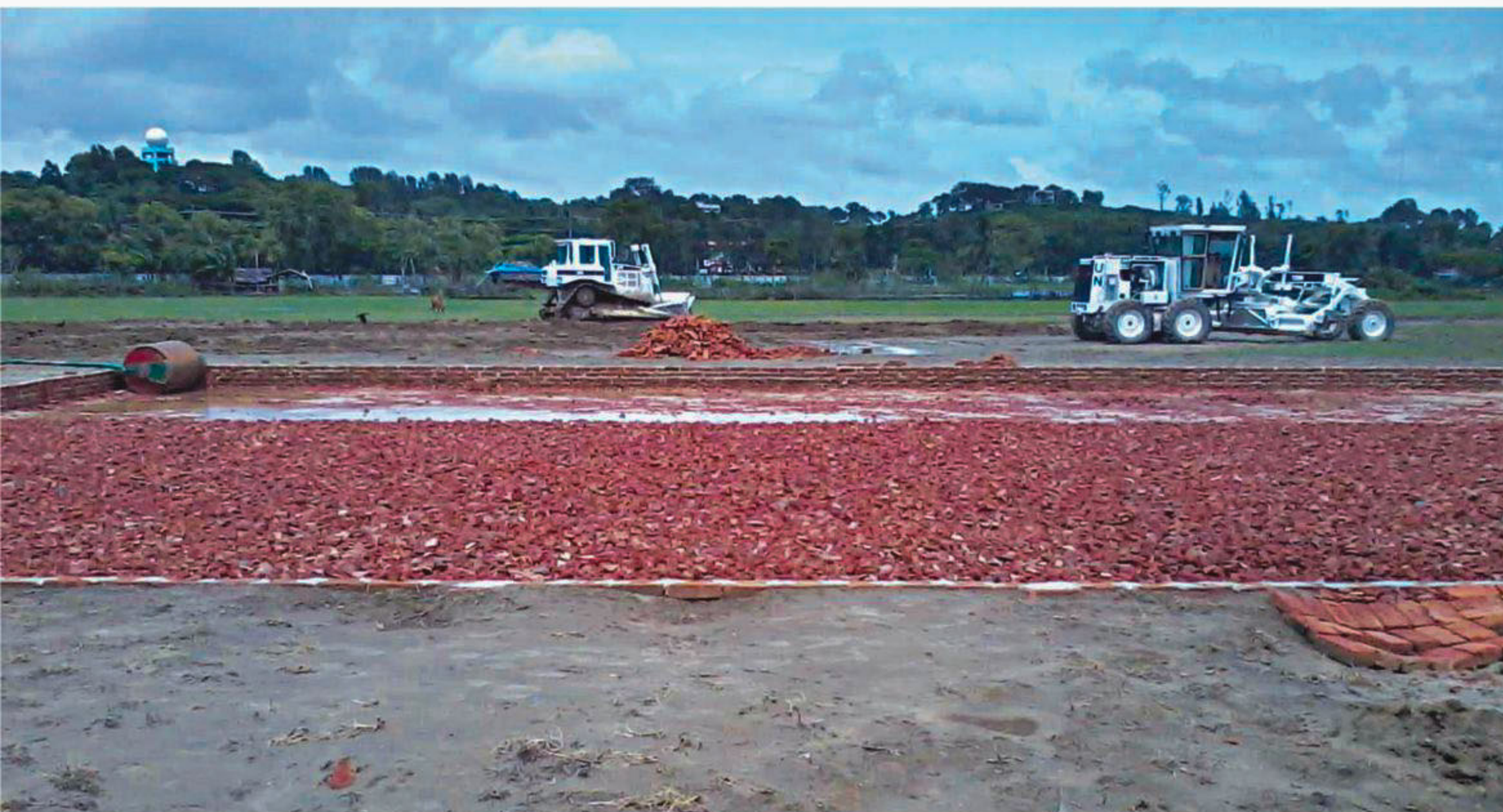
The construction work of the proposed venue for the 2014 ICC T20 Women's World Cup in Cox's Bazar got a real shot in the arm after the Engineering Corps of Bangladesh Army got involved from Monday. The picture taken on Thursday shows the pitch is taking shape to be ready in time for an August inspection.
