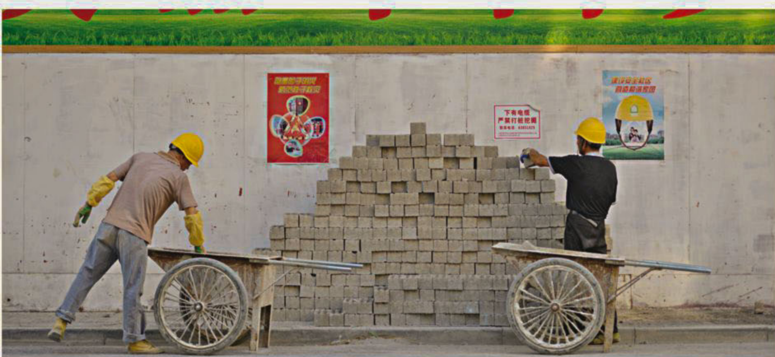
Workers in Shanghai unload bricks under a sign that reads "Beautiful Chinese Dream" in Chinese characters.
