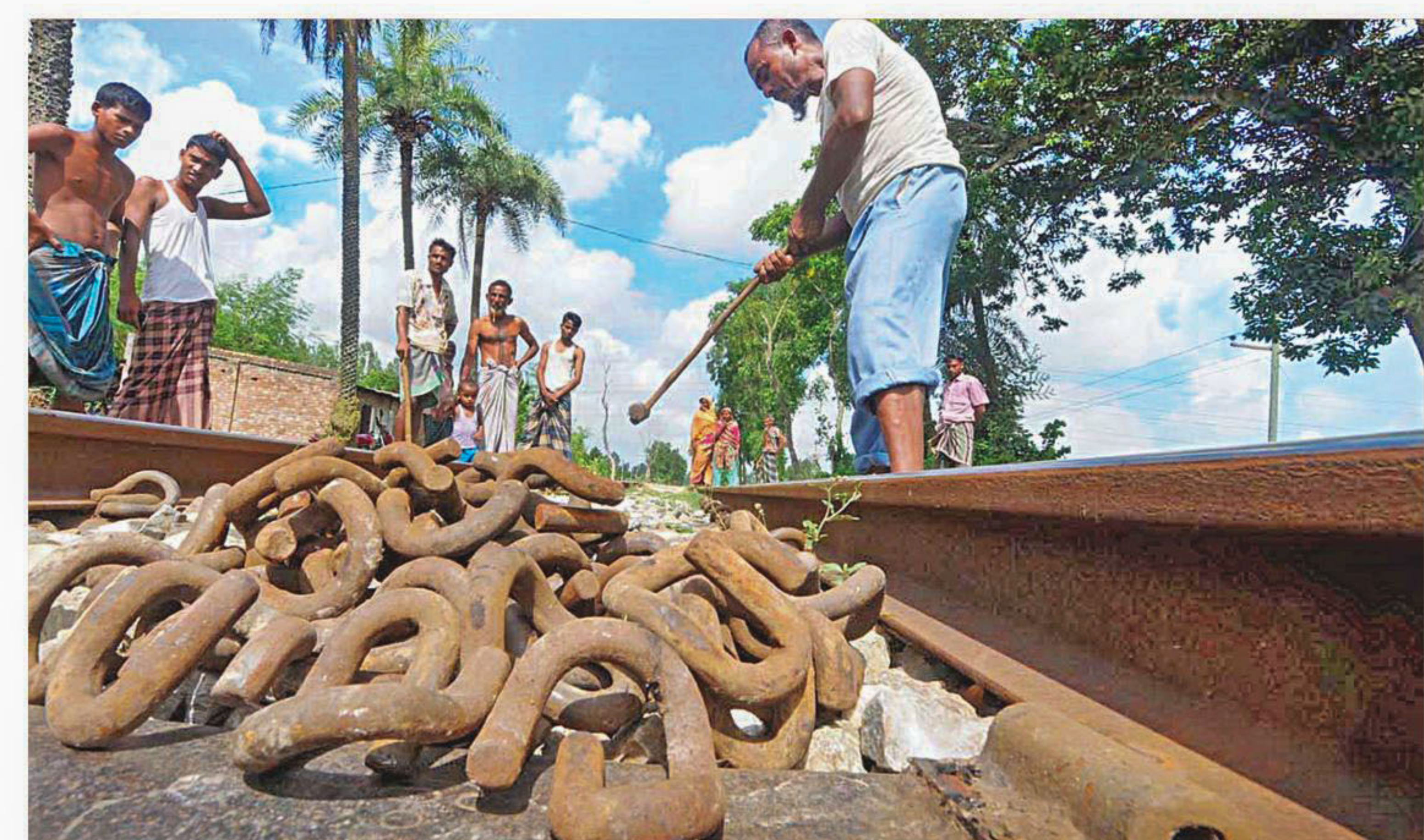
Workers try to reinstall the sleeper clips criminals removed from around 300 metre stretch of rail lines in Dighi area of Bogra town early yesterday. PHOTO: FOCUS BANGLA
