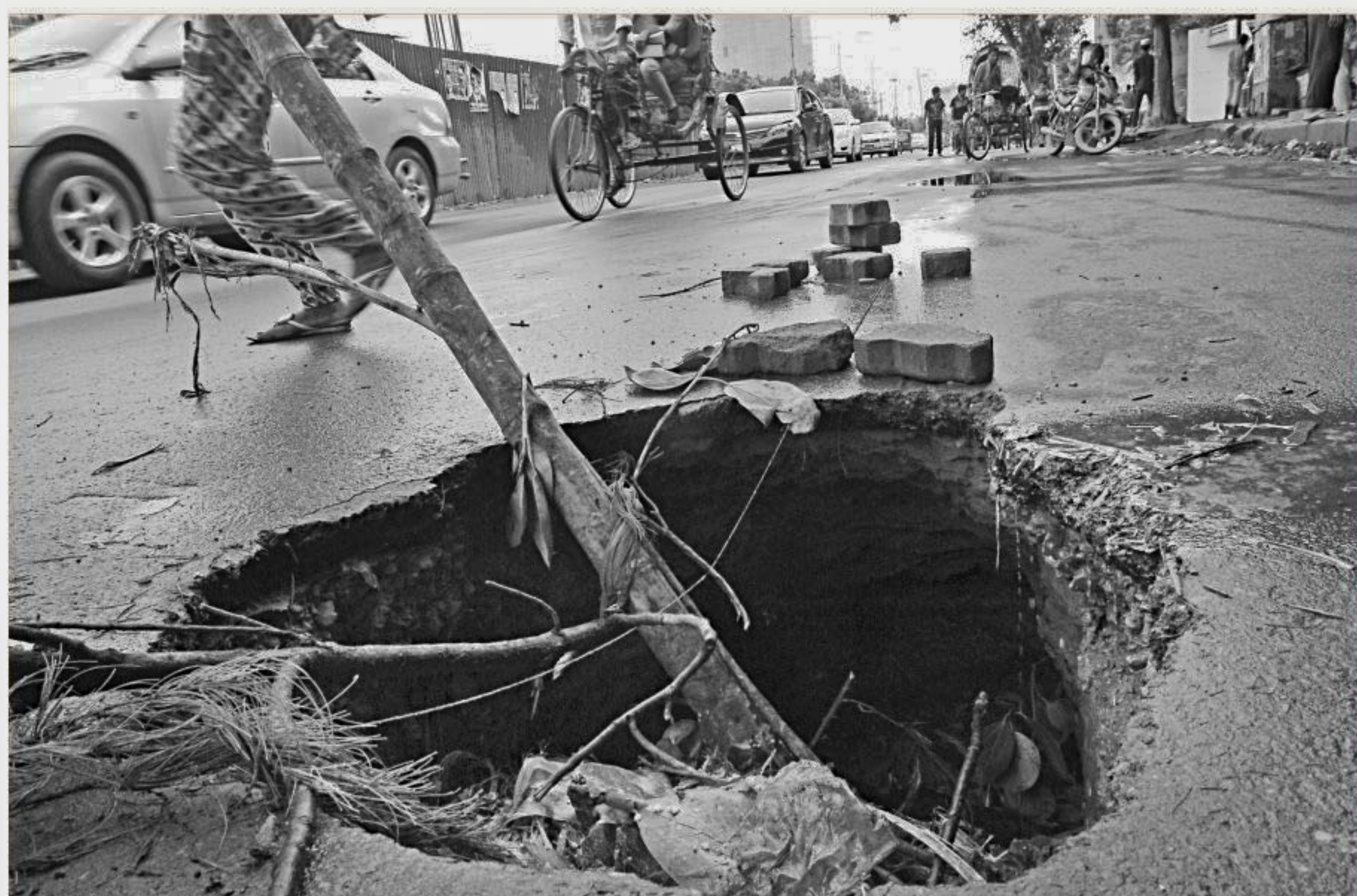
The road before the capital's Bangladesh Film Development Corporation caved in while only a branch serves as a warning for oncoming traffic, leaving the risk of an accident anytime. The photo was taken yesterday. PHOTO: PALASH KHAN
