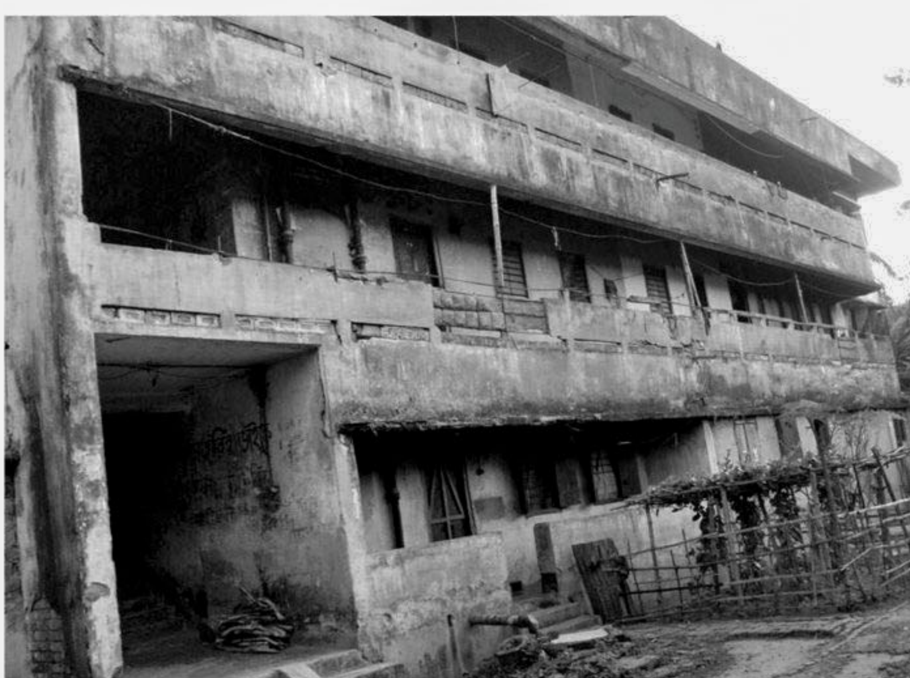
Authorities on Tuesday vacated this building, used earlier as residential quarters by families of 18 employees of Mobarakganj Sugar Mills in Kaliganj upazila under Jhenidah district, declaring it unfit for use.
