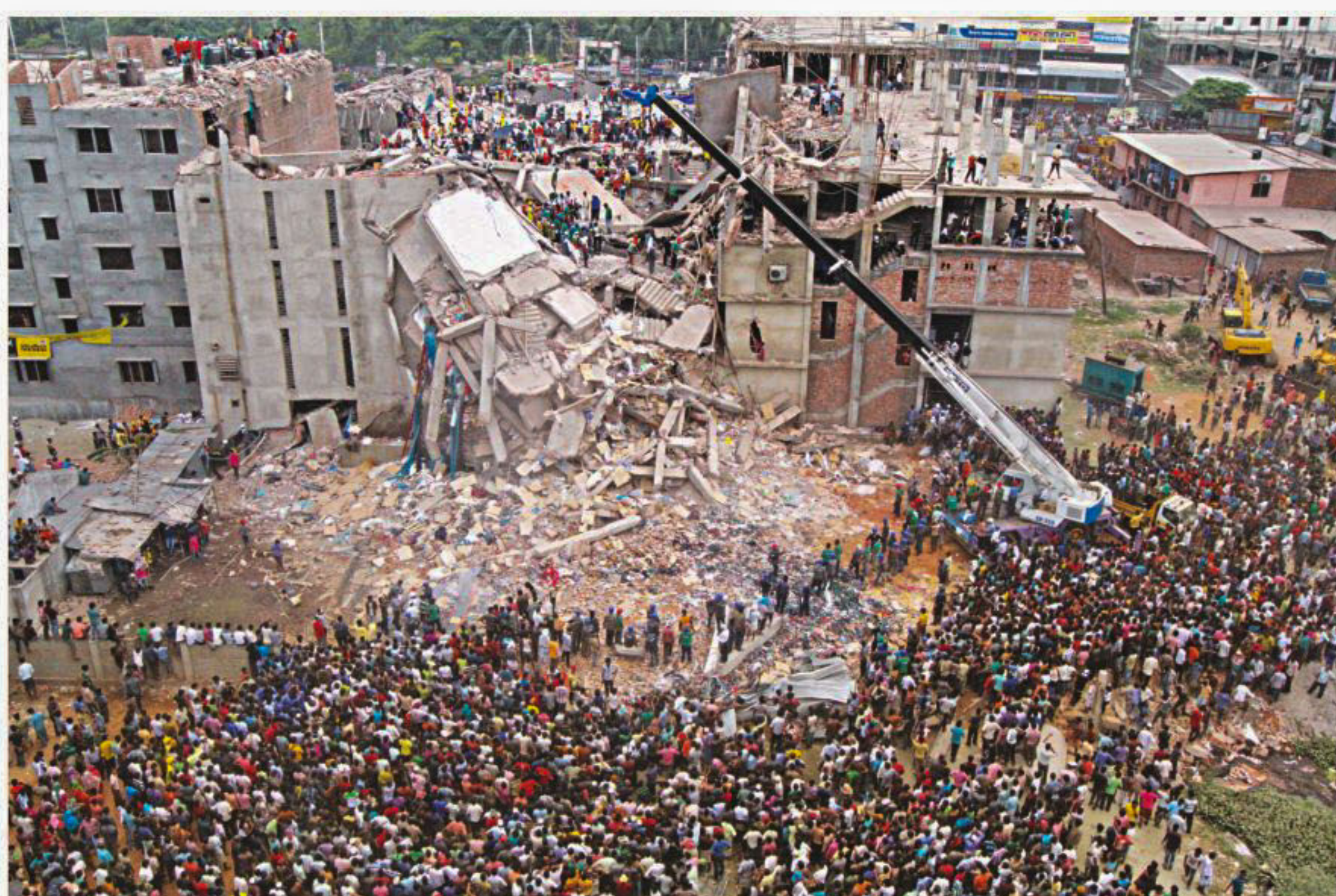
A crane is being used to clear the rubble of the collapsed Rana Plaza in Savar on April 25. STAR/FILE
