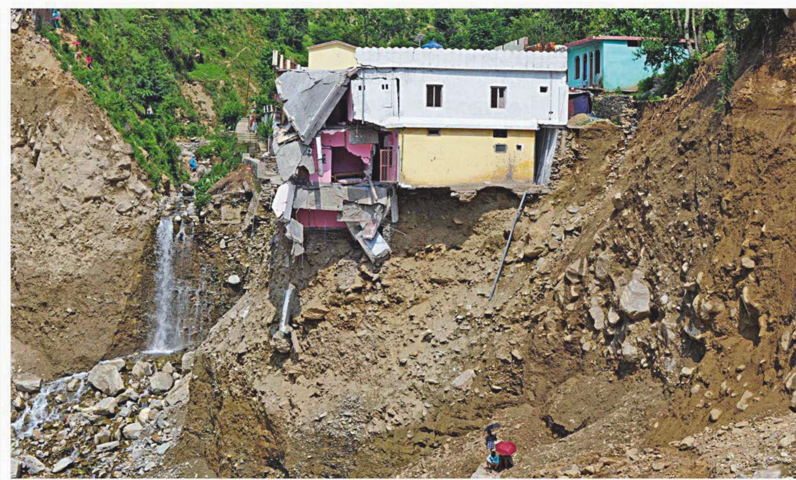
A damaged house perches on the mountainside alongside the Mandakini river at Silli, in the flood affected area of northern Uttarakhand state on Monday. Construction along river banks will be banned in a devastated north Indian state amid concerns unchecked development fuelled last month's flash floods and landslides that killed thousands, the state's top official said yesterday.
