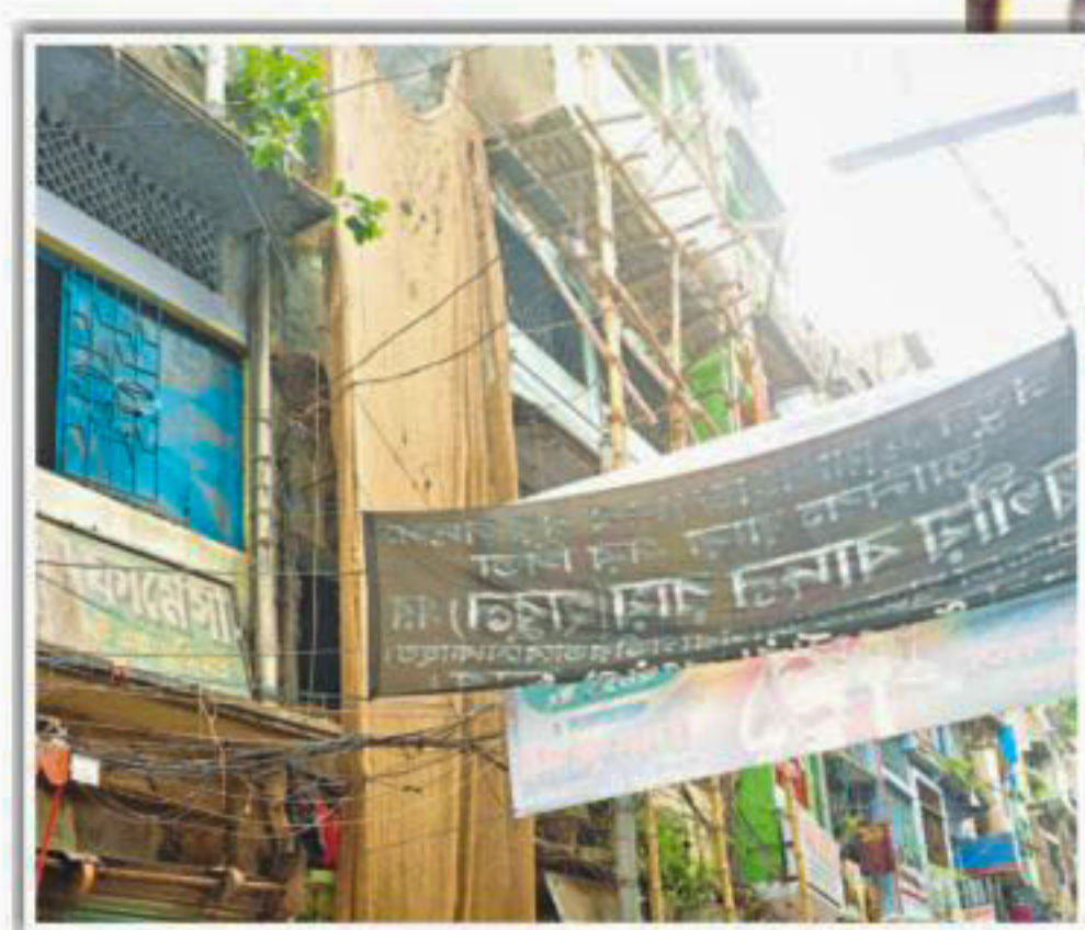
A heritage building during demolition on the capital's Shankhari Lane last month. The government listed 142 holdings along the lane for preservation as heritage sites. Owners of such properties blame the government for not providing the mandated necessary maintenance and restoration support. They have formed a committee demanding freedom to dispose of their structures however they want. Inset, the facade of the building draped in a jute sheet for demolition. PHOTO: STAR
