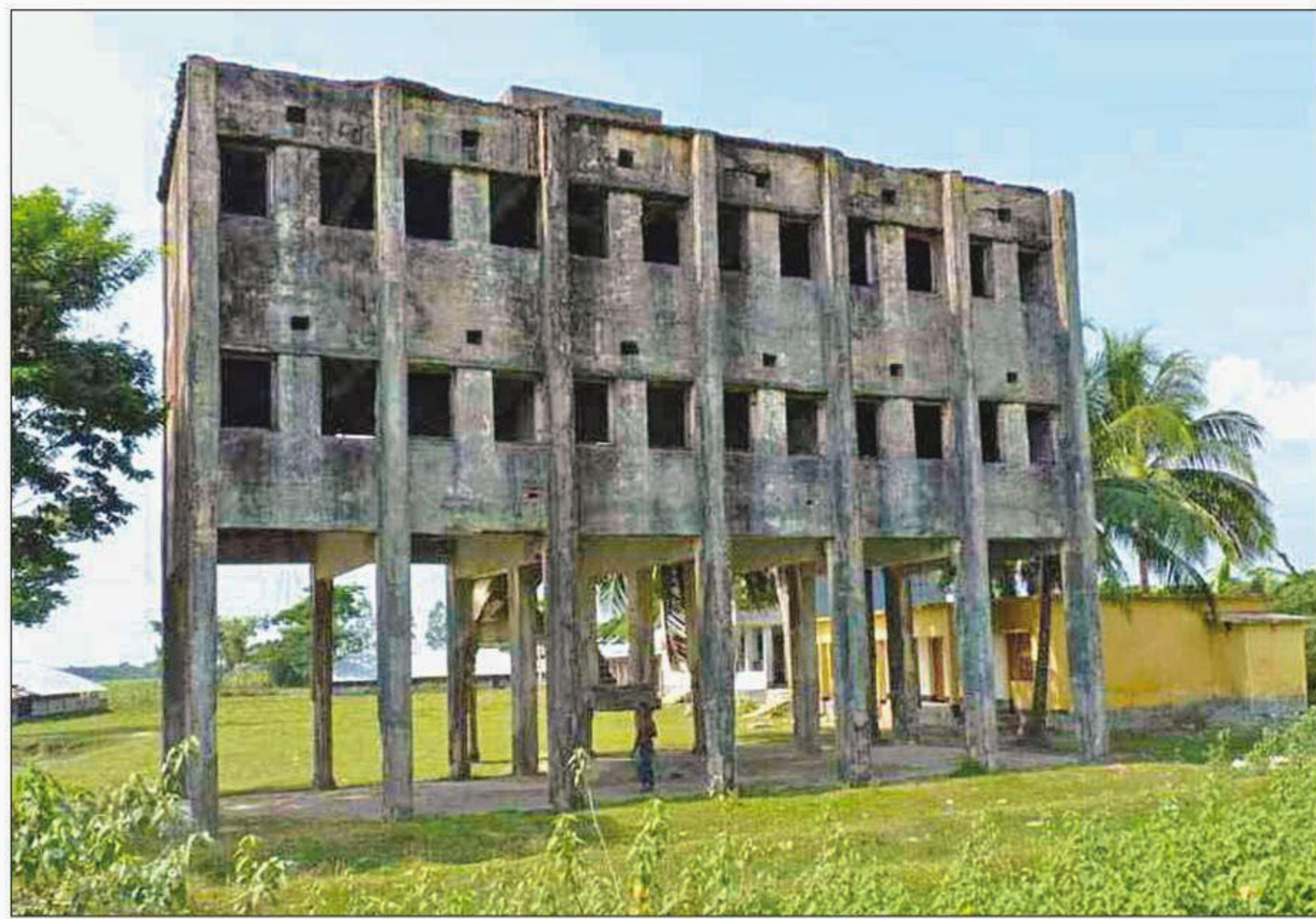
A cyclone shelter in Galachipa upazila of Patuakhali, which has become unusable for a lack of maintenance.
