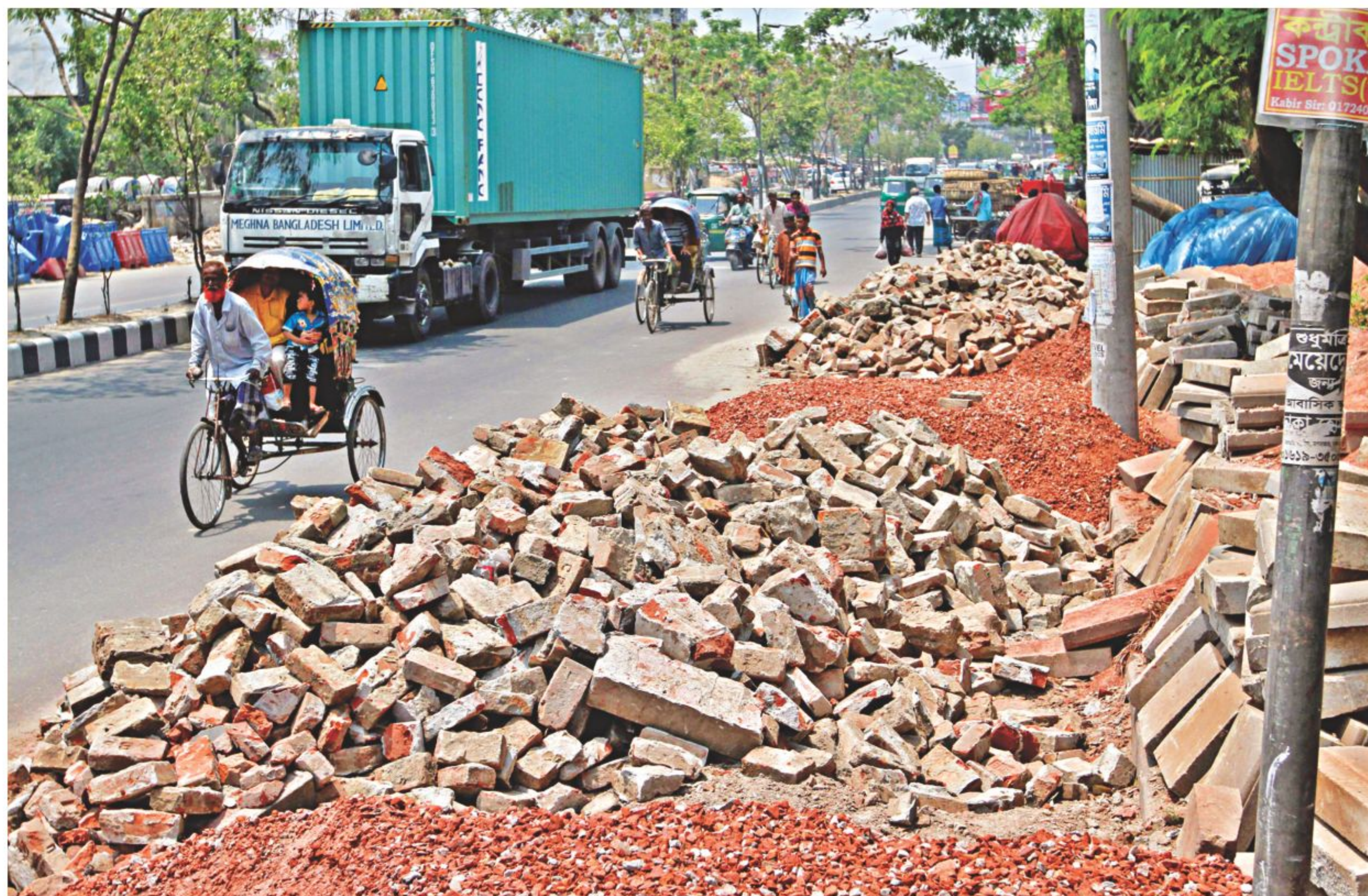
Dhaka South City Corporation blocks a part of Malibagh-Khilgaon Road and the adjacent footpath by dumping broken brick pieces and debris there. The waste materials are from development works carried out on roads and footpaths of Khilgaon, Shajahanpur and Kamalapur in the capital. The photo was taken yesterday.
