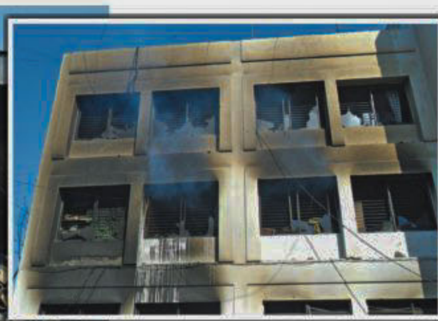
Charred remains of transformers and power supply equipment in Palli Bidyut Office in Kansat area of Chapainawabganj's Shibganj upazila following an arson attack by Jamaat-Shibir activists on Thursday. Inset, the burnt down office. The photos were taken yesterday.
