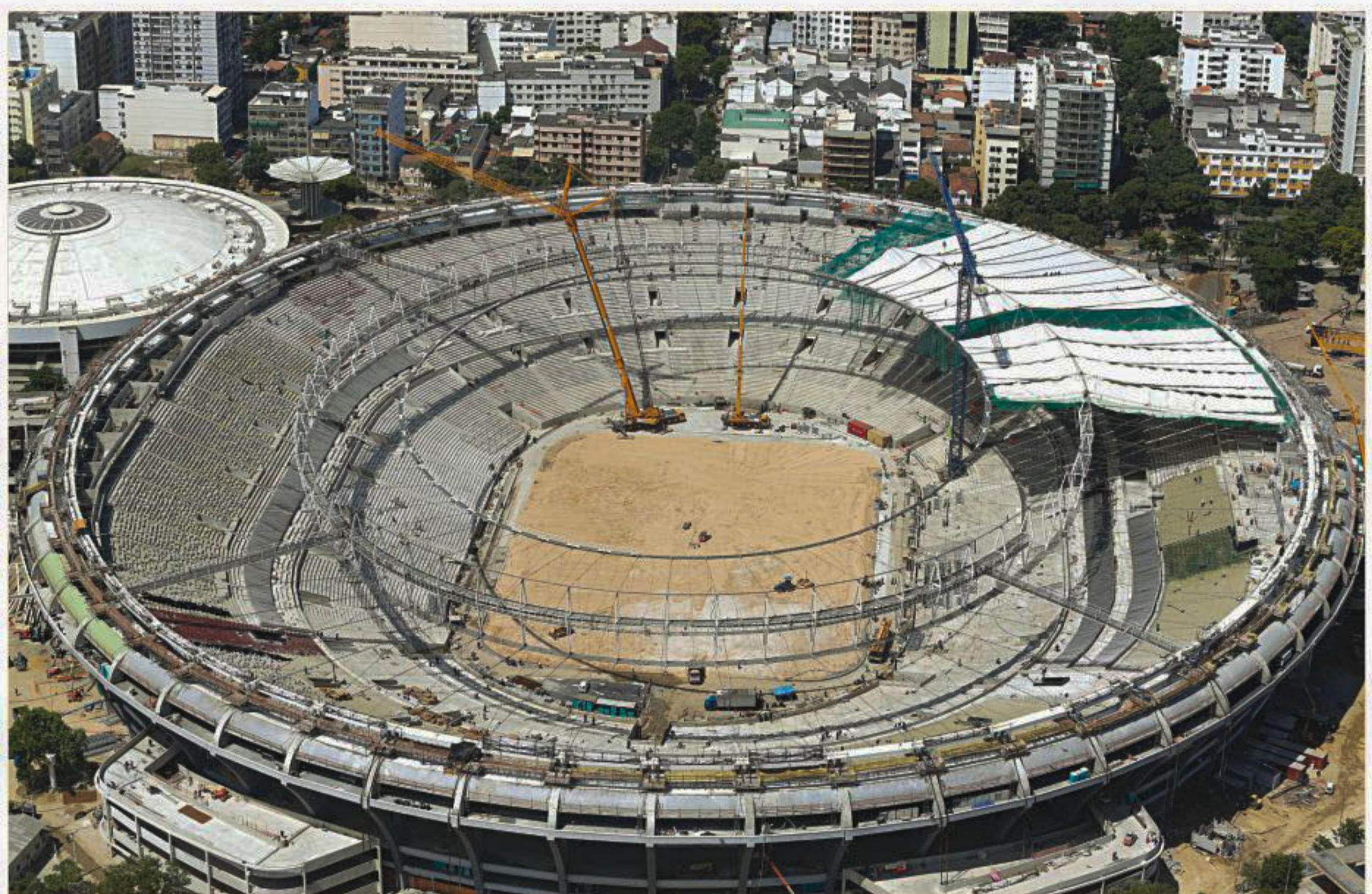
An aerial view shows the roof installation at the Maracana Stadium in Rio which is undergoing renovation for the 2014 World Cup. The stadium will also host games for the 2013 Confederations Cup.
