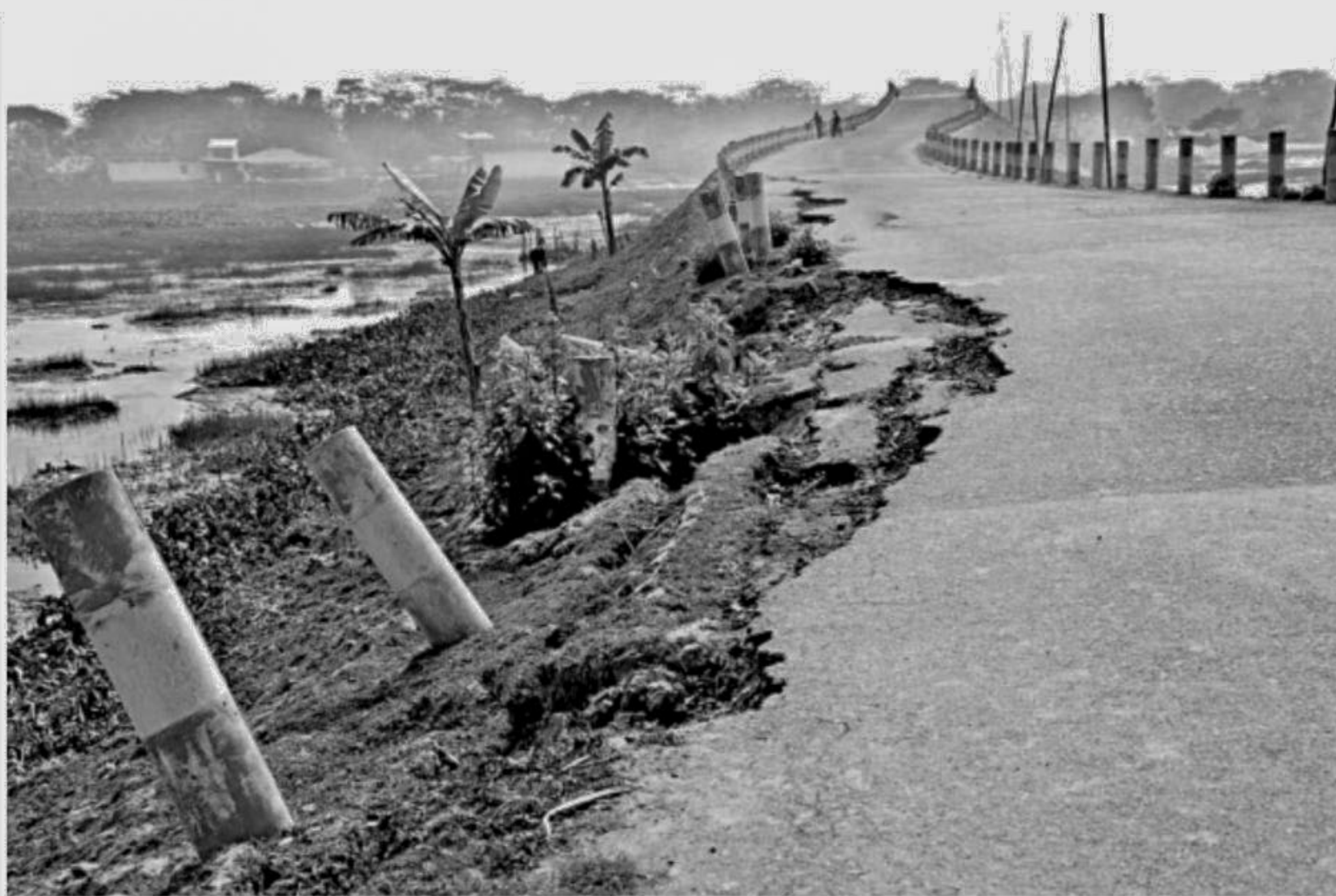
Shayestabad Bridge in Barisal City Corporation area getting damaged within a year of construction, much to the worries of local commuters. Photo shows a portion of the bridge subsiding near the water body.
