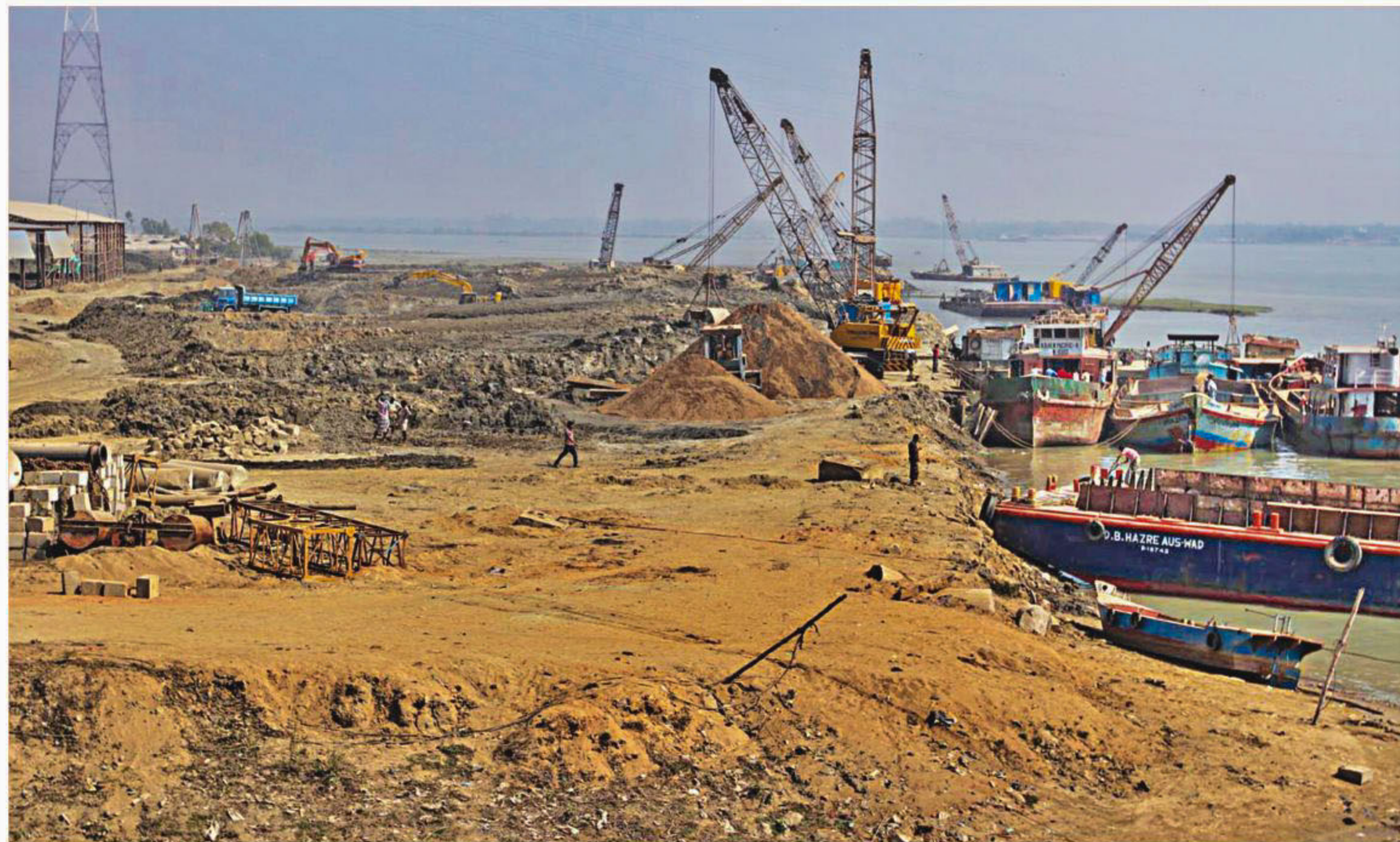
Work is going on in full swing to construct a road along Karnaphuli river, from Sadarghat to Kalurghat in Chittagong city, along with a walkway. The road is being constructed as part of Chittagong port's river training project with assistance from Chittagong City Corporation and Chittagong Development Authority. Once complete, the road is expected to act as a recreational facility for the port city's dwellers. The photo was taken recently.
