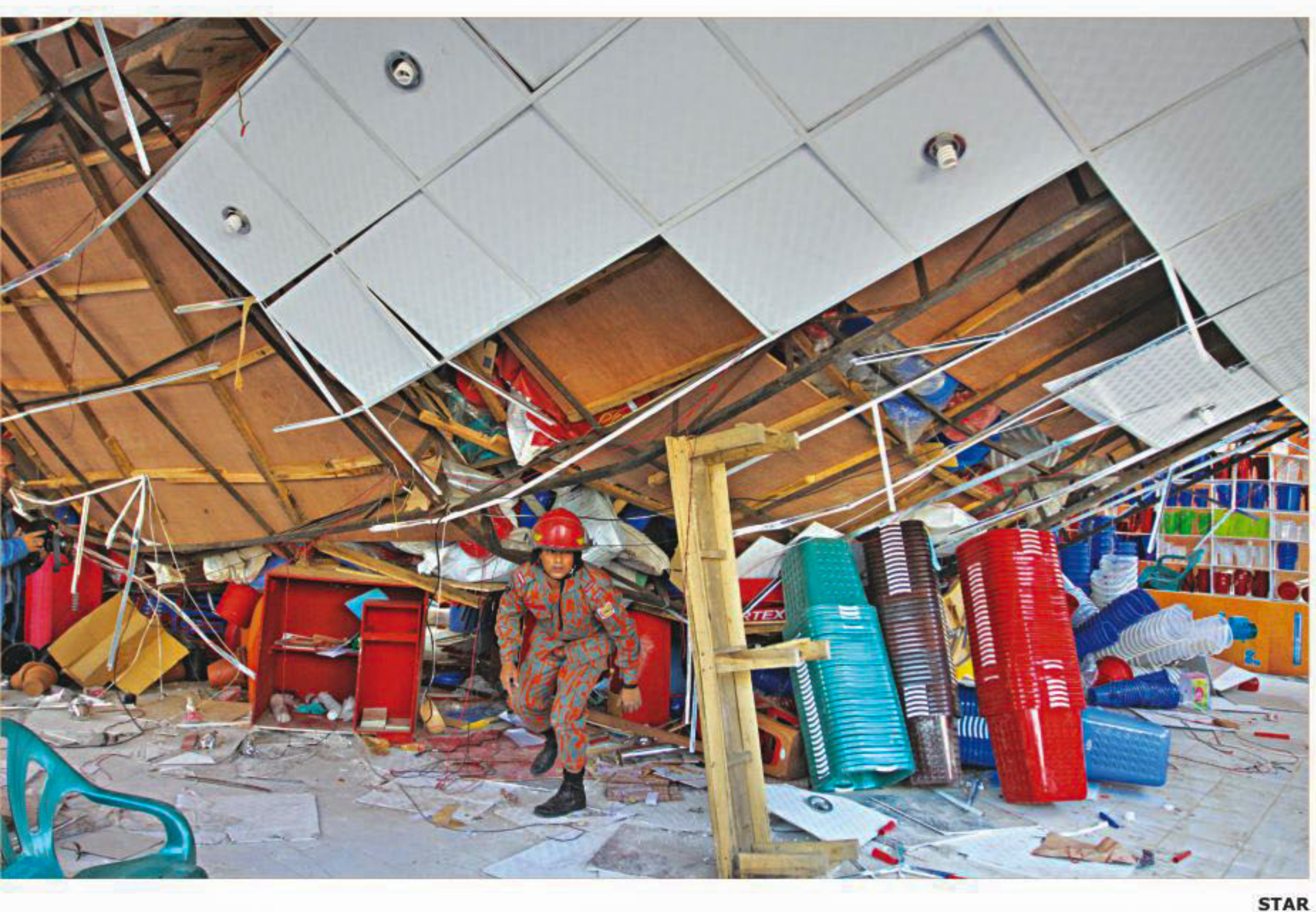
An official of Bangladesh Fire Service and Civil Defence checks out the Partex Plastics pavilion that collapsed yesterday, killing an employee of the company at the Dhaka International Trade Fair. Story on page 20
