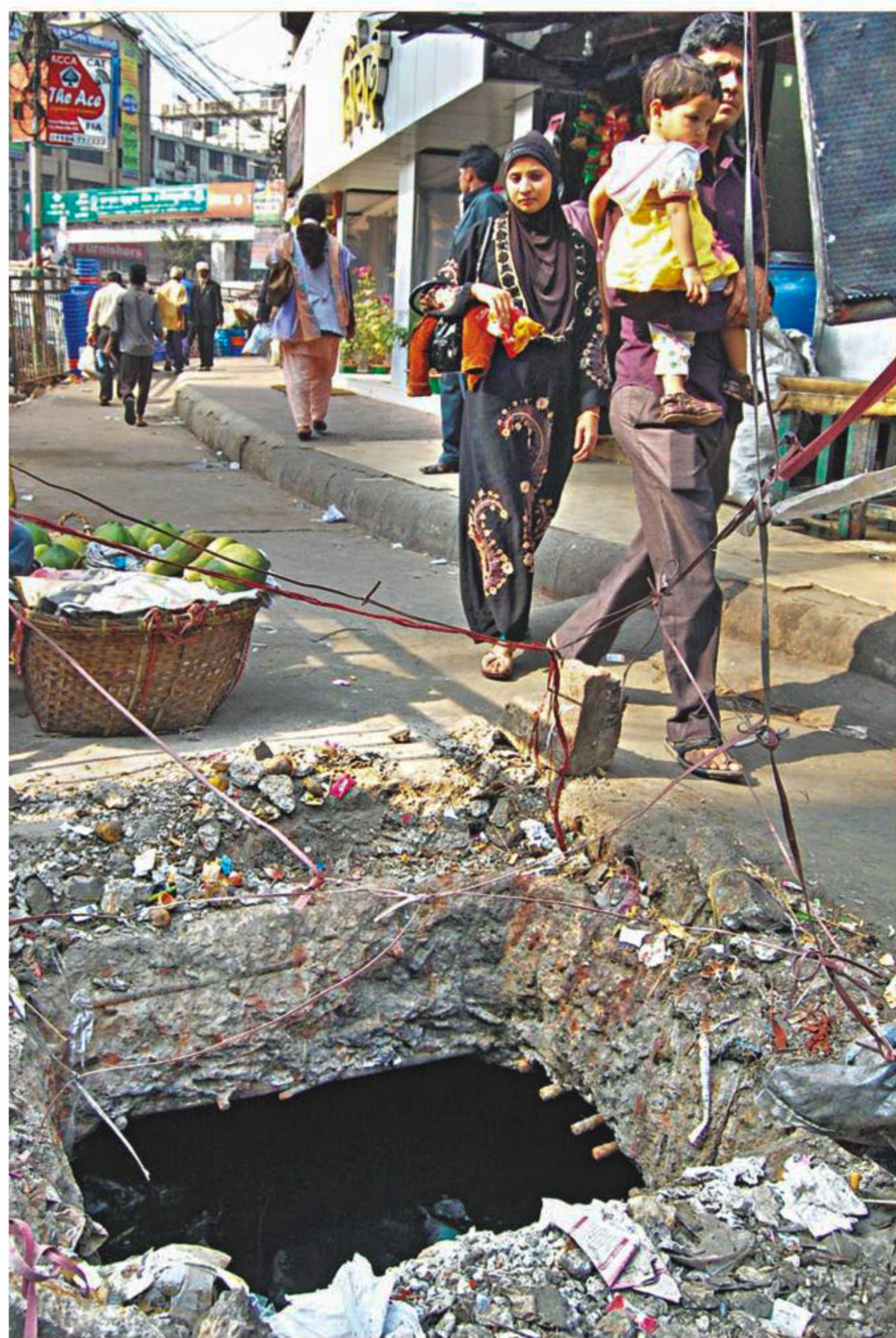
The manhole at GEC intersection in Chittagong city, which is missing its cover for the last 10 days, fails to grab the attention of the authorities concerned. The photo was taken on Friday.
