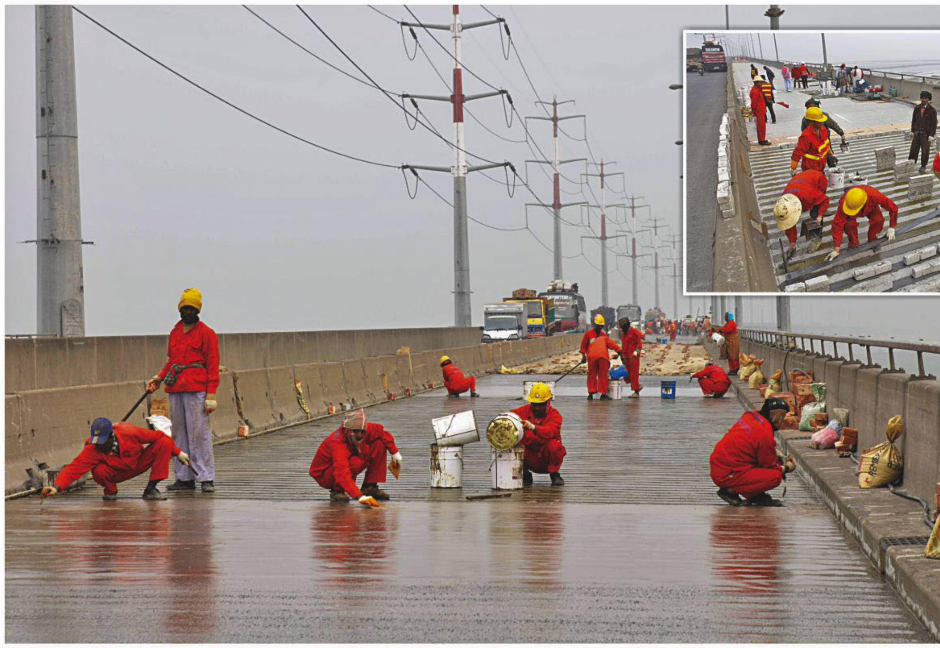
Workers applying epoxy, a type of glue, on the deck of the Bangabandhu Multipurpose Bridge to repair its cracks. Inset, Workers pasting a chemical on the cracks. The photos were taken recently.
