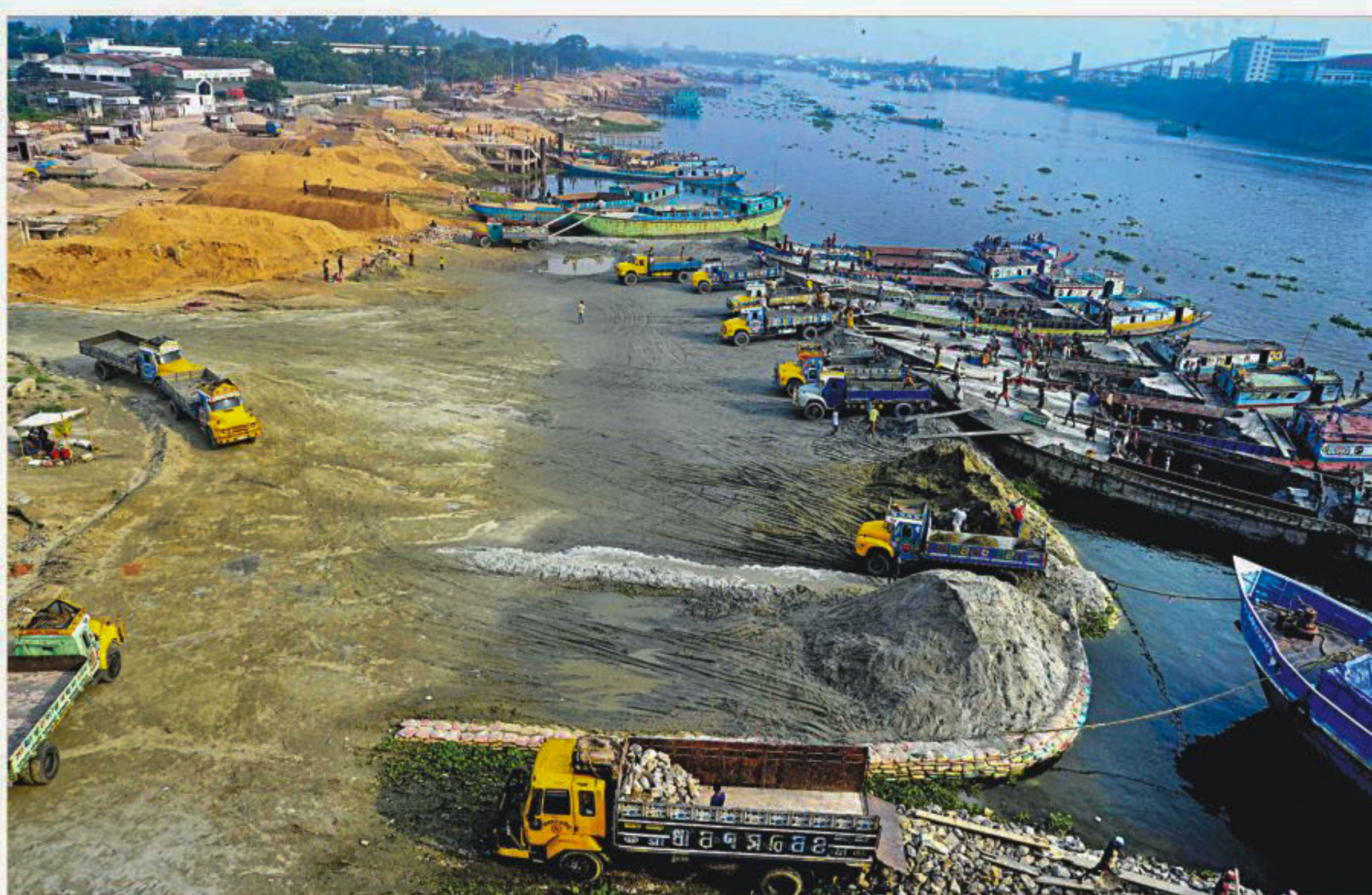
Sand traders, under the very nose of the administration, continue to encroach upon the Shitalakkhya by dumping construction materials illegally. As a result, the river has been narrowed down almost to its half near Kanchpur bridge in Naryanganj. The photo was taken recently.
