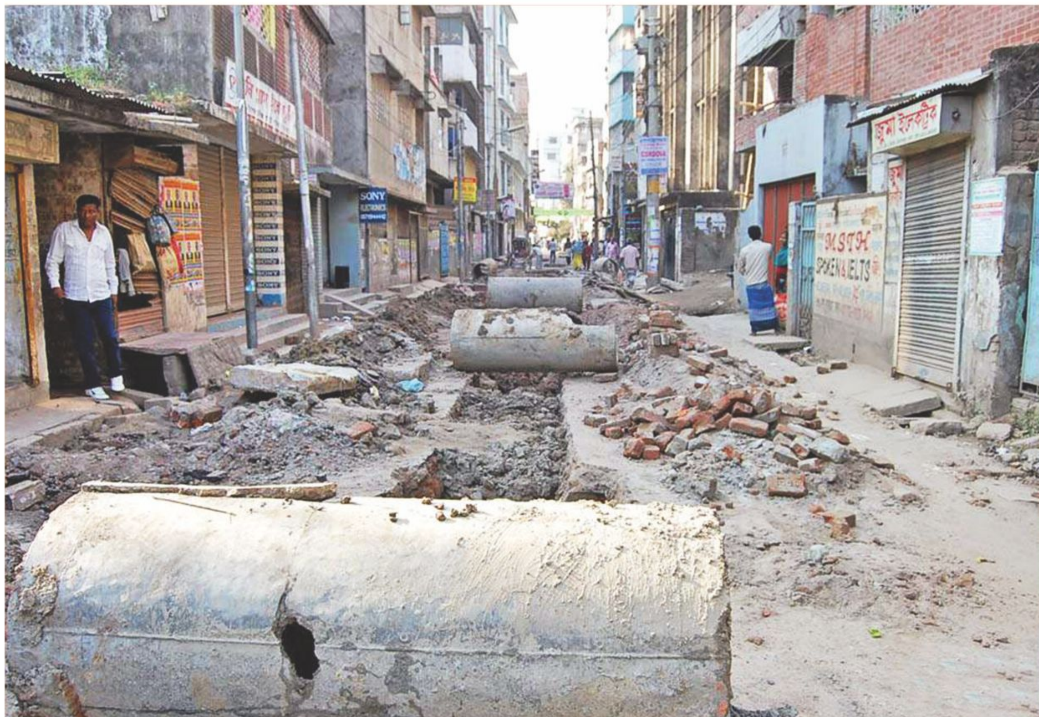
Sewerage pipes, bricks and mud have been rendering a road in front of Dhaka South City Corporation's Tilpapara office in the capital's Khilgaon useless for a long time. Delay by the contractors tasked with the sewerage development work is causing sufferings to the area's inhabitants. The photo was taken yesterday.
