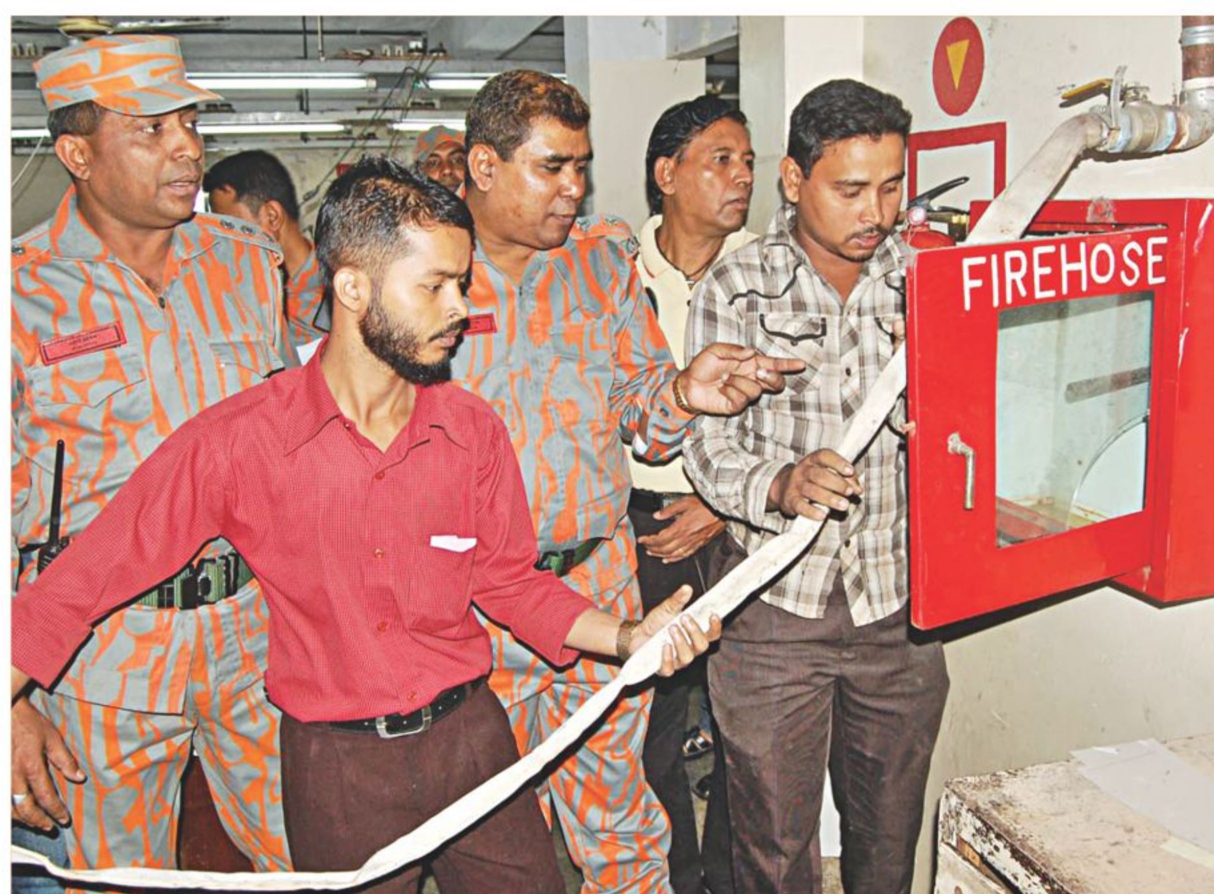
Fire Service and Civil Defence personnel inspect a fire hose in a garment factory in Dewan Haat of Chittagong city yesterday against the backdrop of a devastating fire in a garment factory of Ashulia on November 24 which claimed 111 workers' lives.
