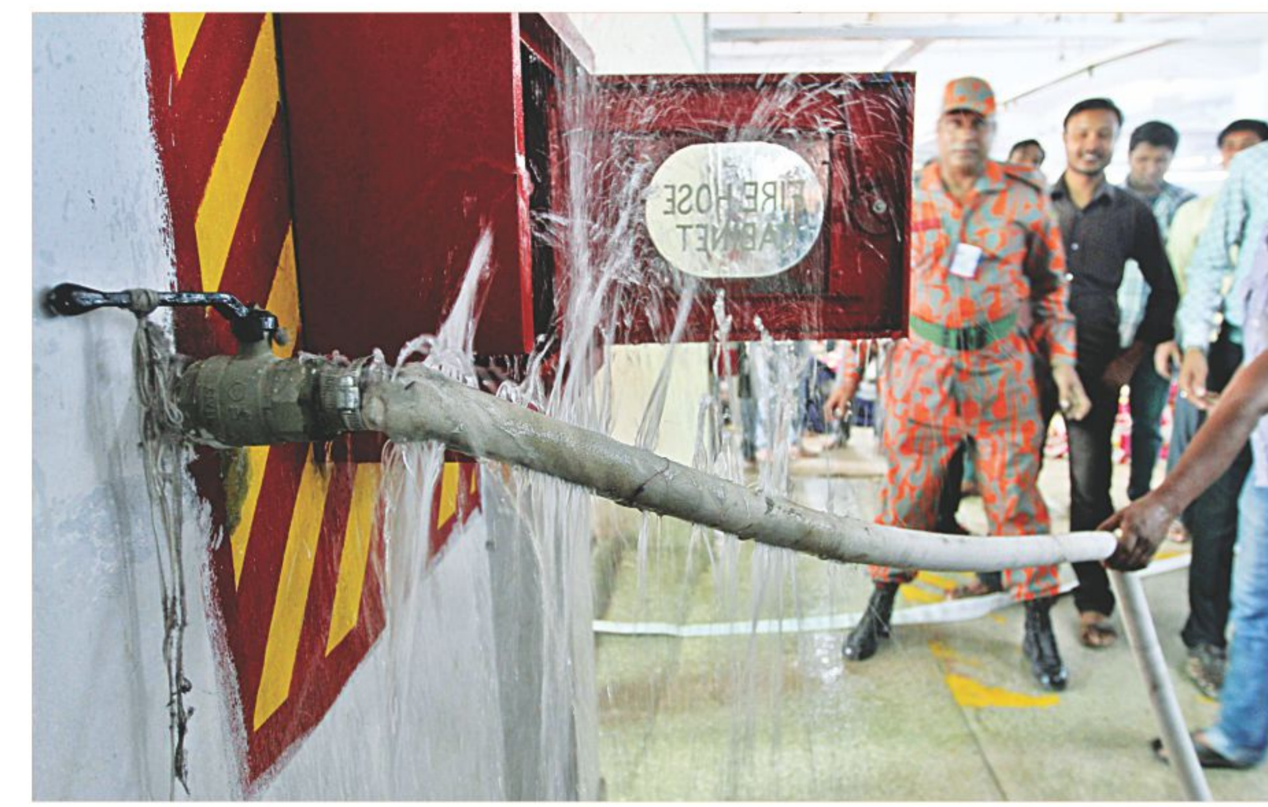
The fire brigade inspects different garment factories in Ashulia to check their fire safety equipment yesterday, a week after 111 people died in the Tazreen Fashions blaze. The photo shows a fire-dousing hose of a factory leaking badly.
