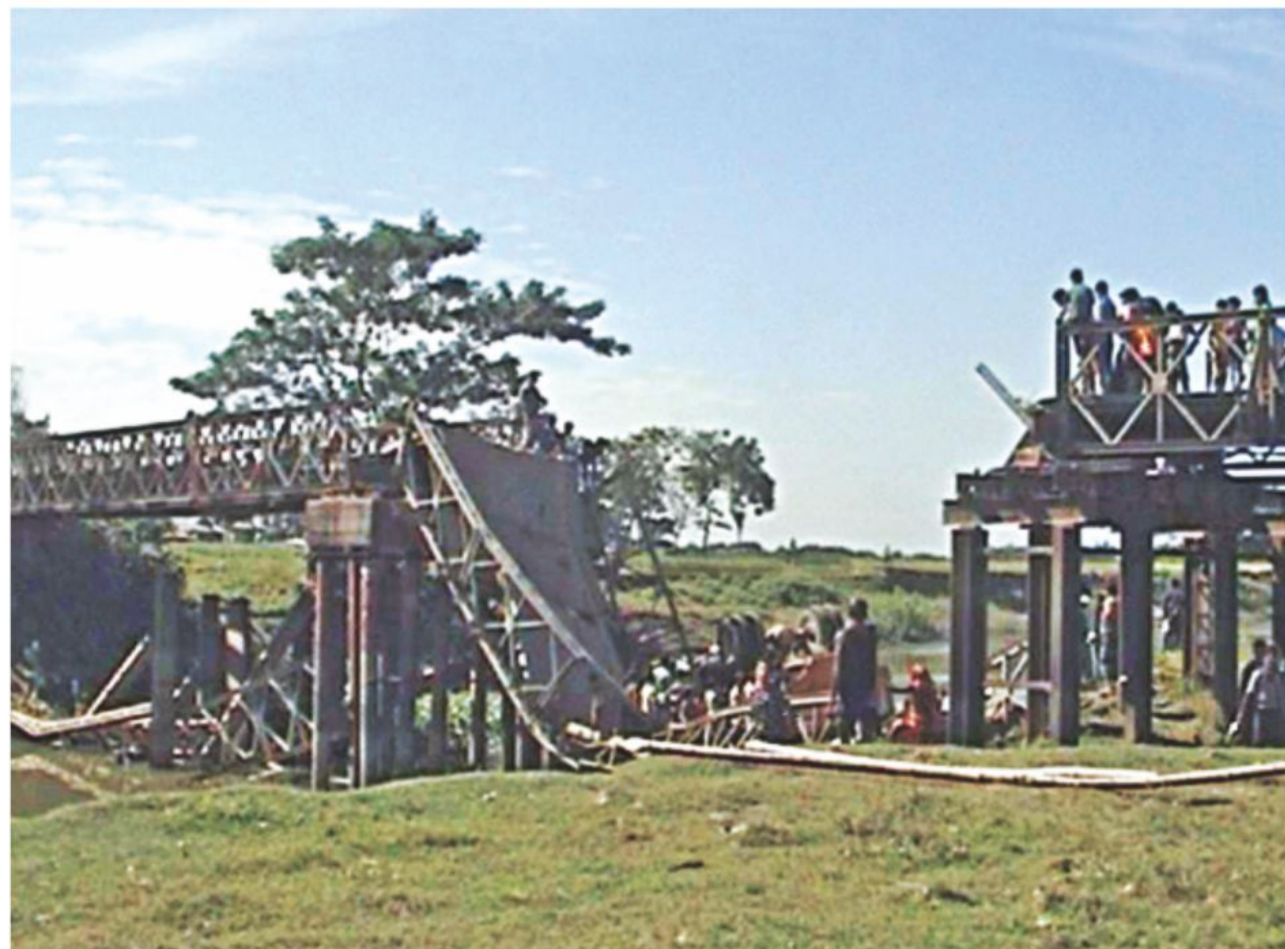
PHOTO: STAR This bailey bridge on Durgapur-Mymensingh road at Rajabazar in Purbodhala upazila under Netrakona district collapsed under the pressure of a clay-laden truck yesterday morning, causing suspension of road communication with the district headquarters.
