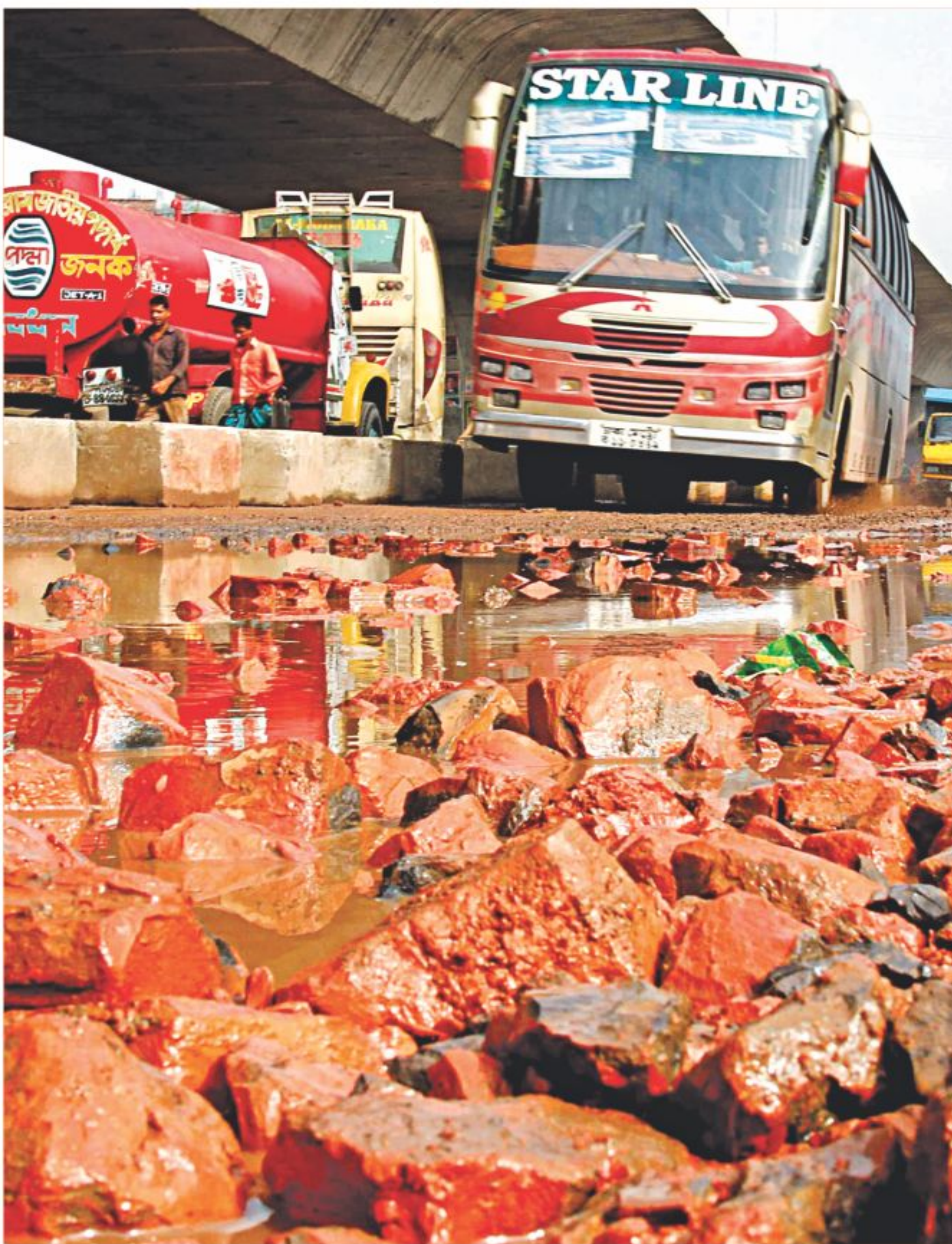
The entire carriageway of a stretch of the capital's Sayedabad road, which was temporarily repaired just ahead of Eid-ul-Azha, has returned to bad shape again. The photo was taken near Sayedabad level-crossing yesterday. PHOTO: STAR
