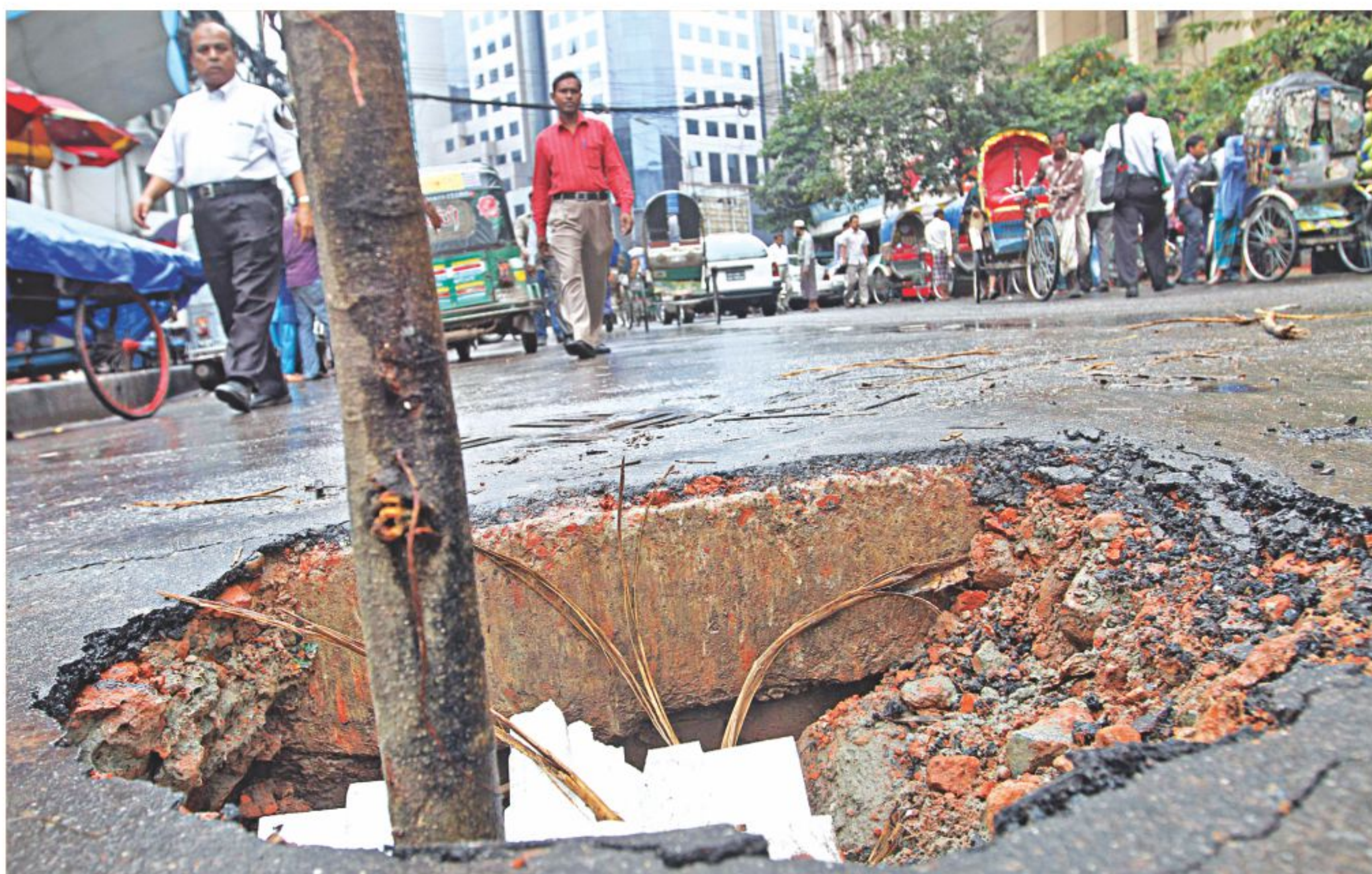
A crater caused by caved in road near the roundabout in front of the Board of Investment causes hazards for vehicles in the capital's Motijheel area. The photo was taken yesterday.
