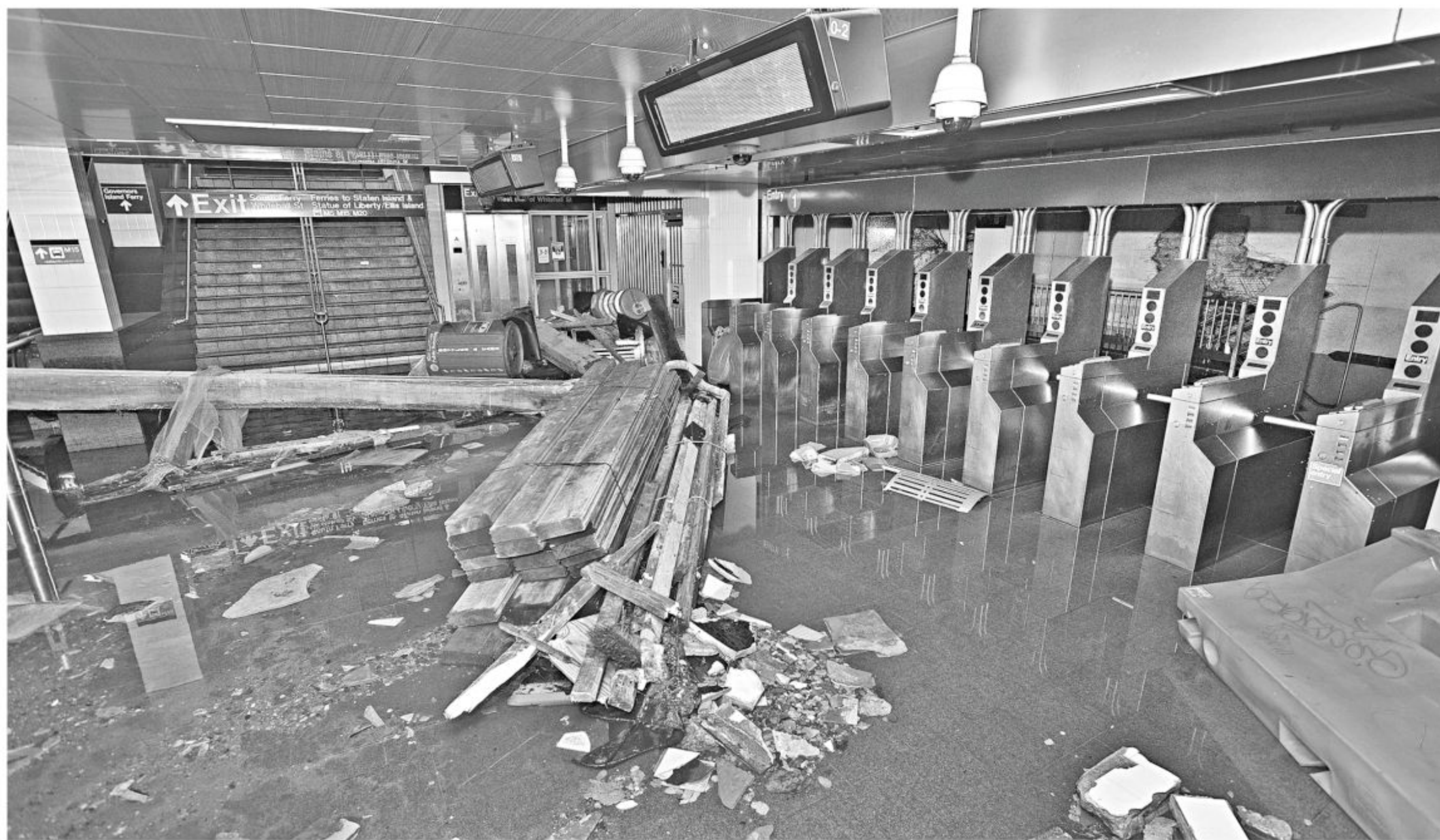
PHOTO: AFP This image obtained from the Metropolitan Transportation Authority of the State of New York shows the South Ferry subway station in New York after it was flooded by seawater during Hurricane Sandy's rampage on Tuesday. The storm carved a trail of devastation across New York City and New Jersey killing more than 55 people as millions remained without power.
