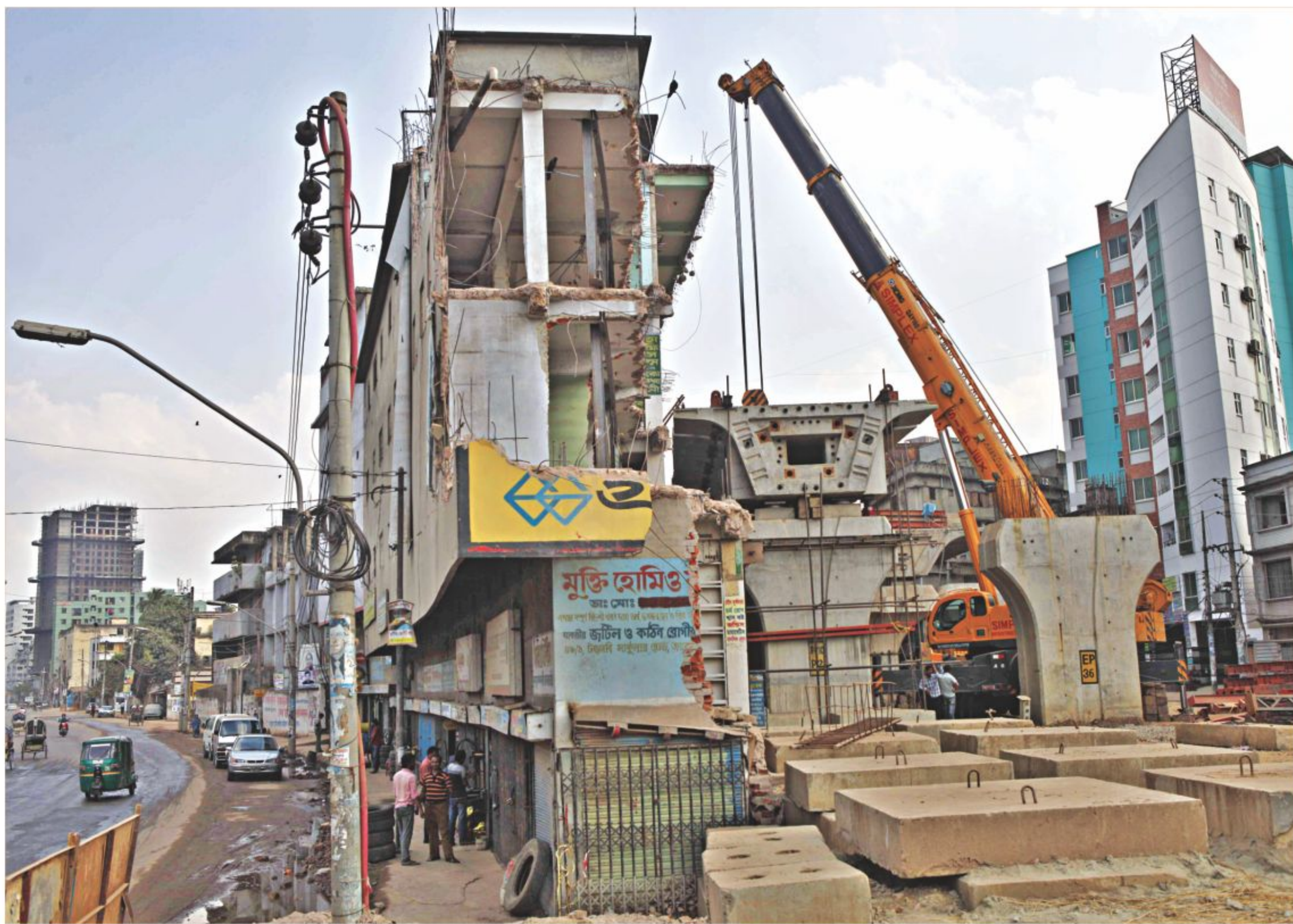
To construct the Jatrabari-Gulistan flyover, one third of this market on Toyenbee Circular Road in the capital has been torn down. However, shop owners continue to use the torn-down building at a risk to their lives. The photo was taken on Tuesday. PHOTO: RASHED SHUMON
