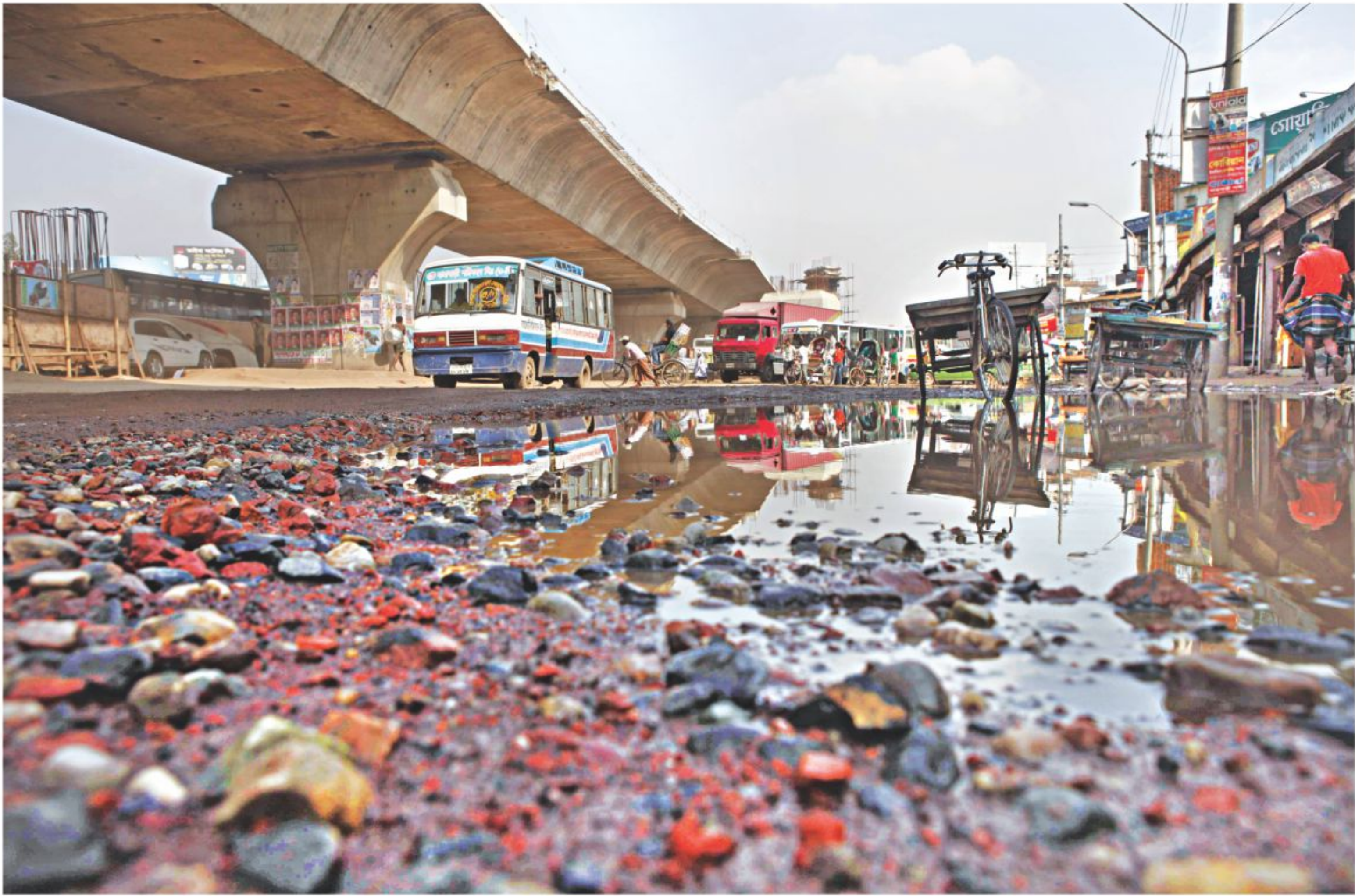
The Dhaka-Chittagong highway in the capital's Jatrabari has long been in bad shape. Whenever it rains, water accumulates in the potholes that have developed on the road owing to a lack of repair and maintenance. The photo was shot on Friday. PHOTO: RASHED SHUMON
