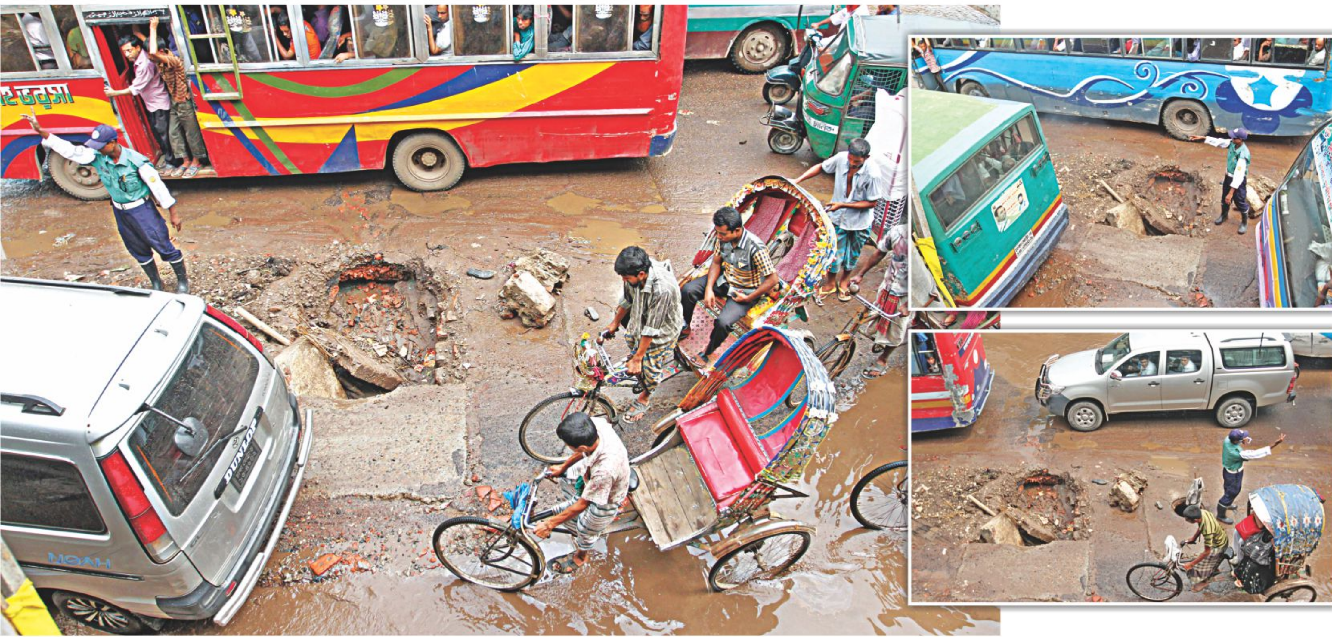
These recent photos taken in front of the city corporation market in Dayaganj area of the capital show the sorry state of two manholes in the middle of the road. One is without a lid and the other is damaged. This was hindering vehicular movement on the busy road so badly that a traffic policeman was deployed to warn motorists of the danger. The policeman himself was in danger of being run over or falling into them.
