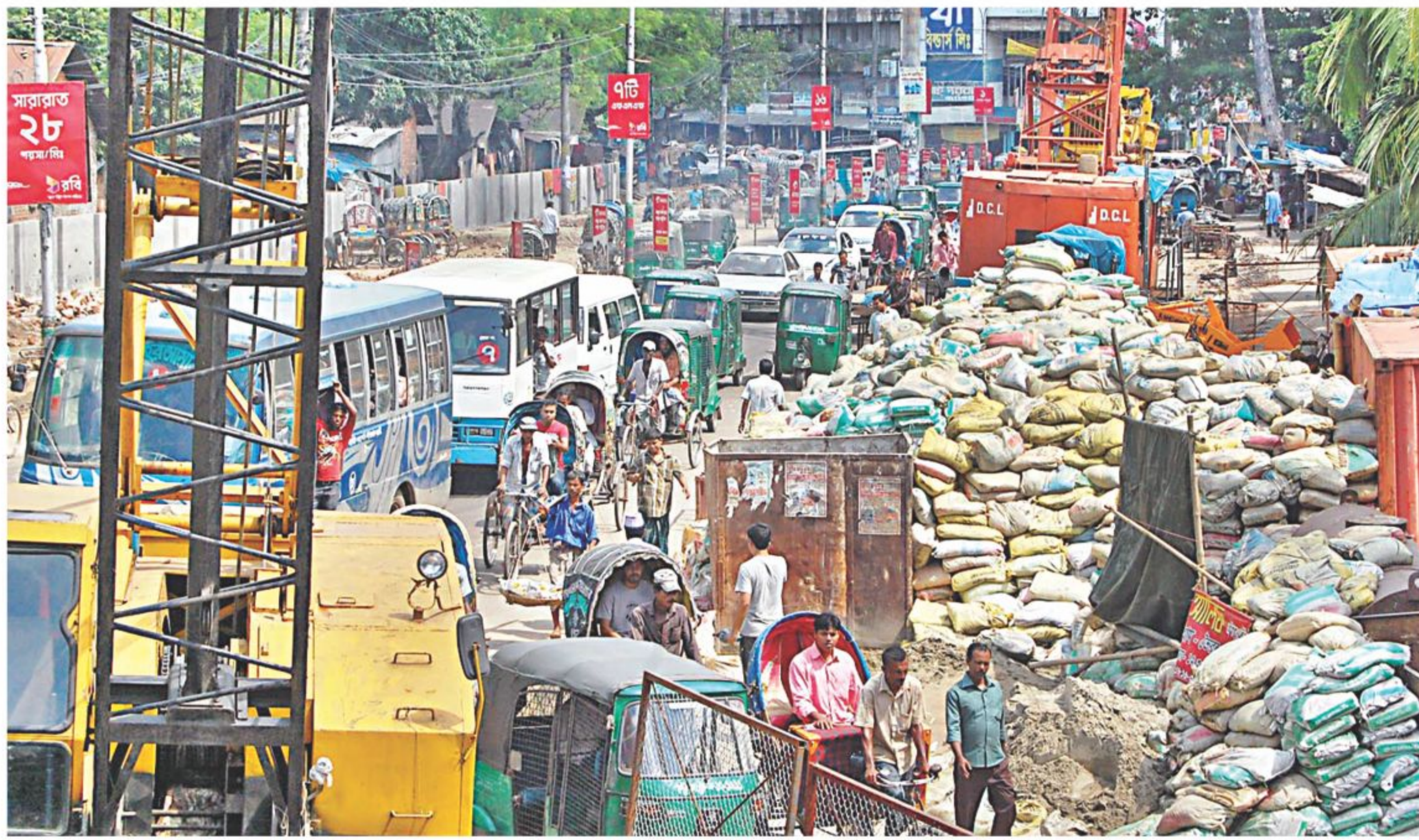
Construction materials of the Kadamtoli flyover in Chittagong city are kept on the pavement and street, disregarding the public suffering it is causing. Day-long traffic congestions have become the norm in the area due to such carelessness. PHOTO: PRABIR DAS
