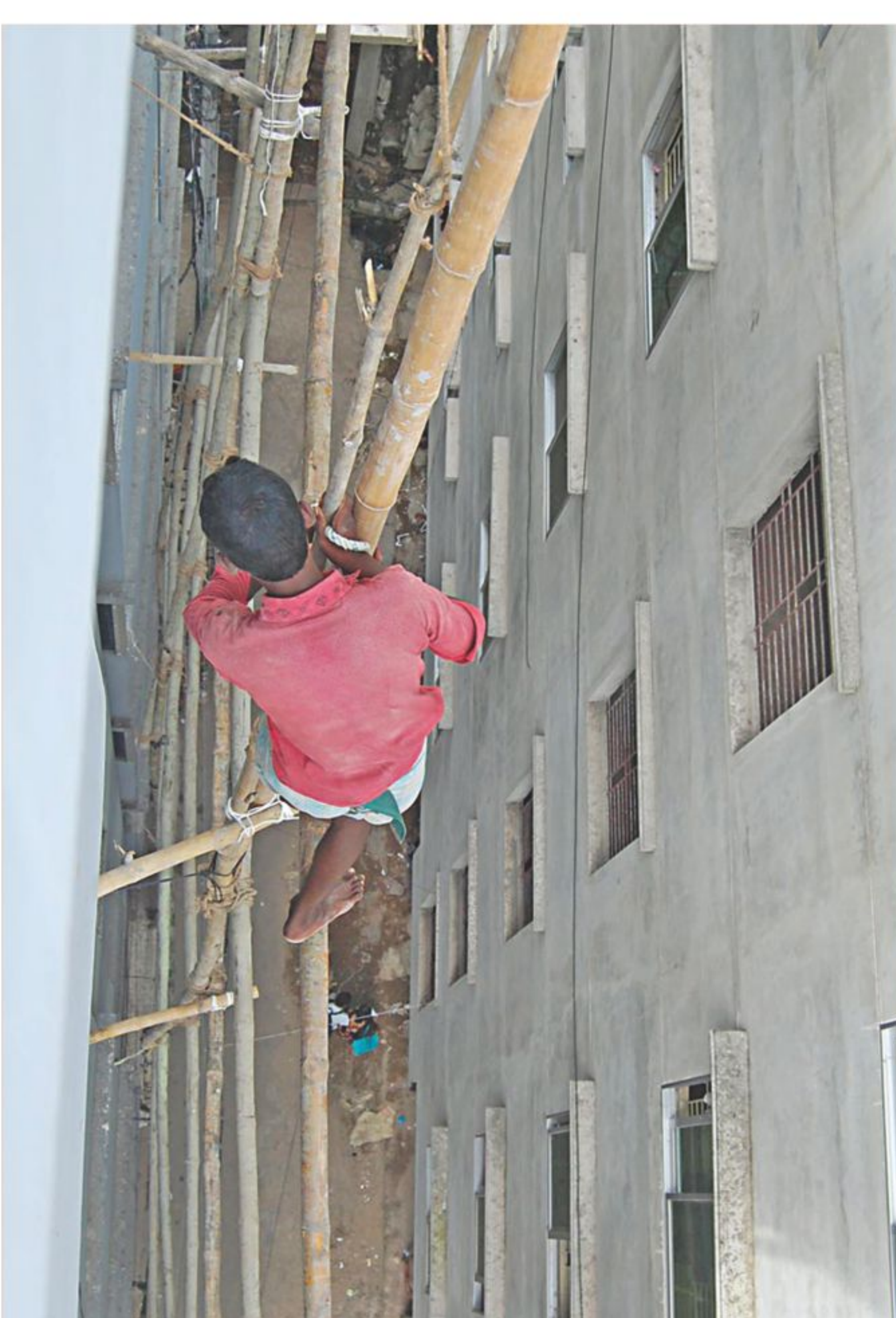
Desperate to make a living, this construction worker braves grave risks to scale a guardrail-less bamboo scaffolding without any safety harness or hard hat in Momin Road in Chittagong city yesterday.
