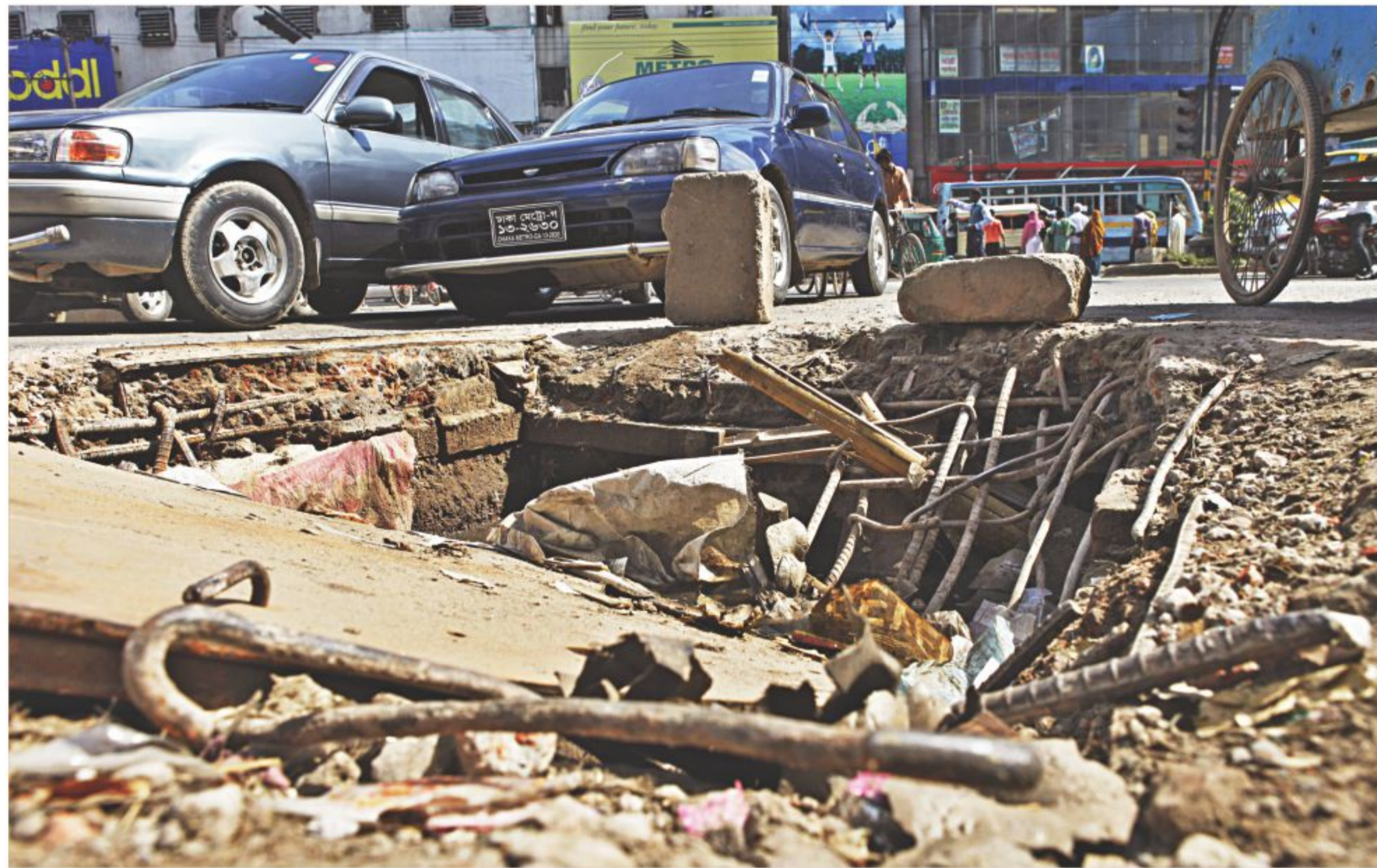
The iron cover on the sewerage line under the capital's Shyamoli link road has collapsed, causing accidents on the road almost every day, while the authorities seem quite indifferent to the situation. The photo was taken yesterday.
