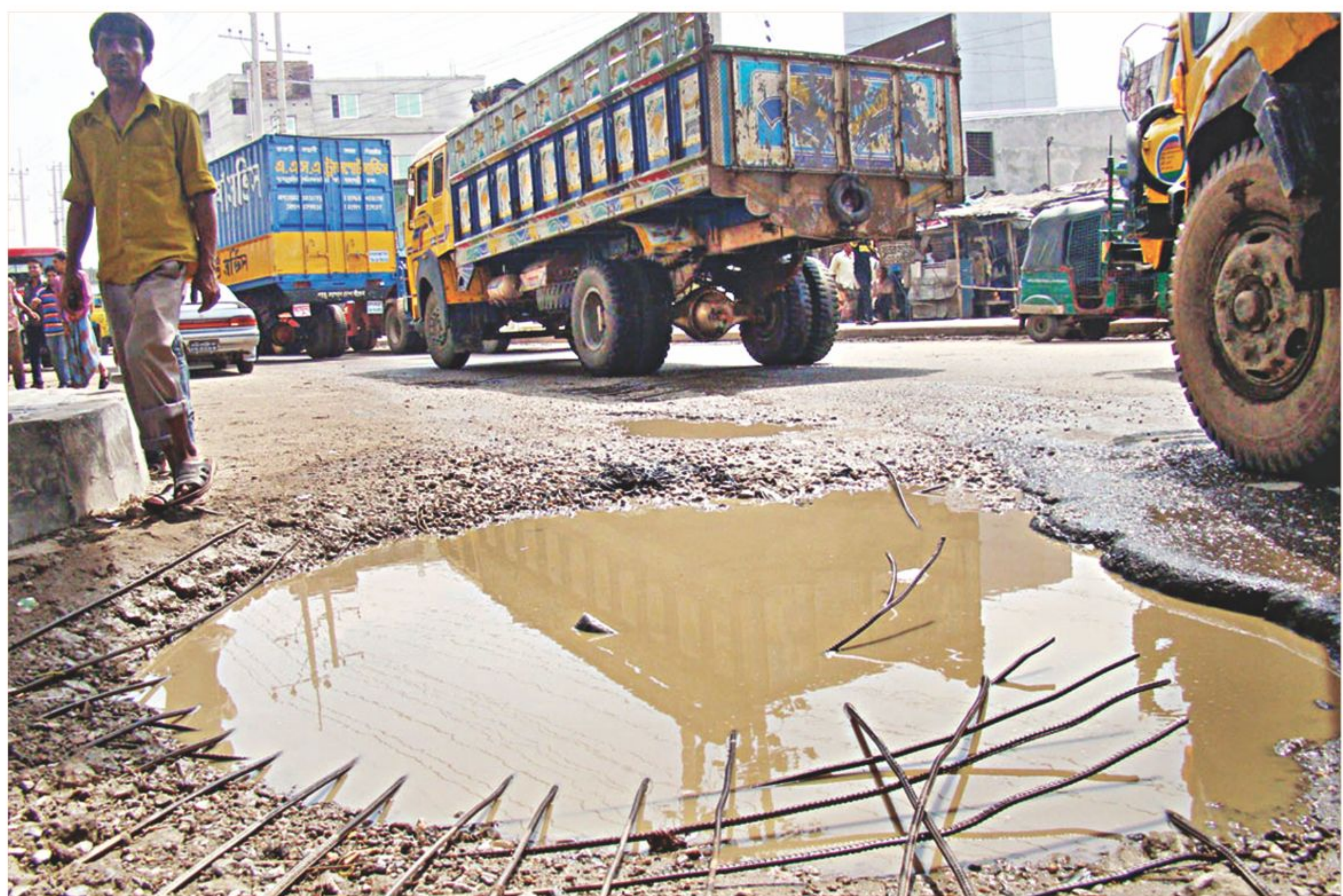
The only road to the new container terminal of Chittagong seaport is filled with craters like this, causing frequent accidents, but the authorities seem to have no care at all.
